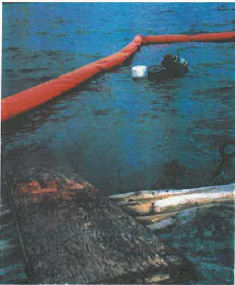
PHOTOGRAPH NO. 10: Diver disconnecting lift buckets inside spill boom prior to barrel removal from water. Note ramp used to roll/lift barrels out of the water up onto the plastic ground sheet.
