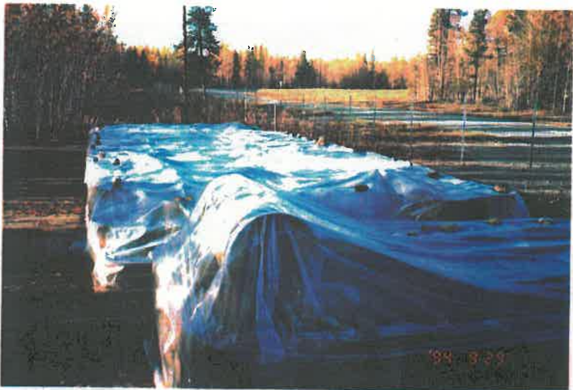
PHOTOGRAPH NO. 14: Barrel storage completed and ready for transport to be recycled or destroyed.
