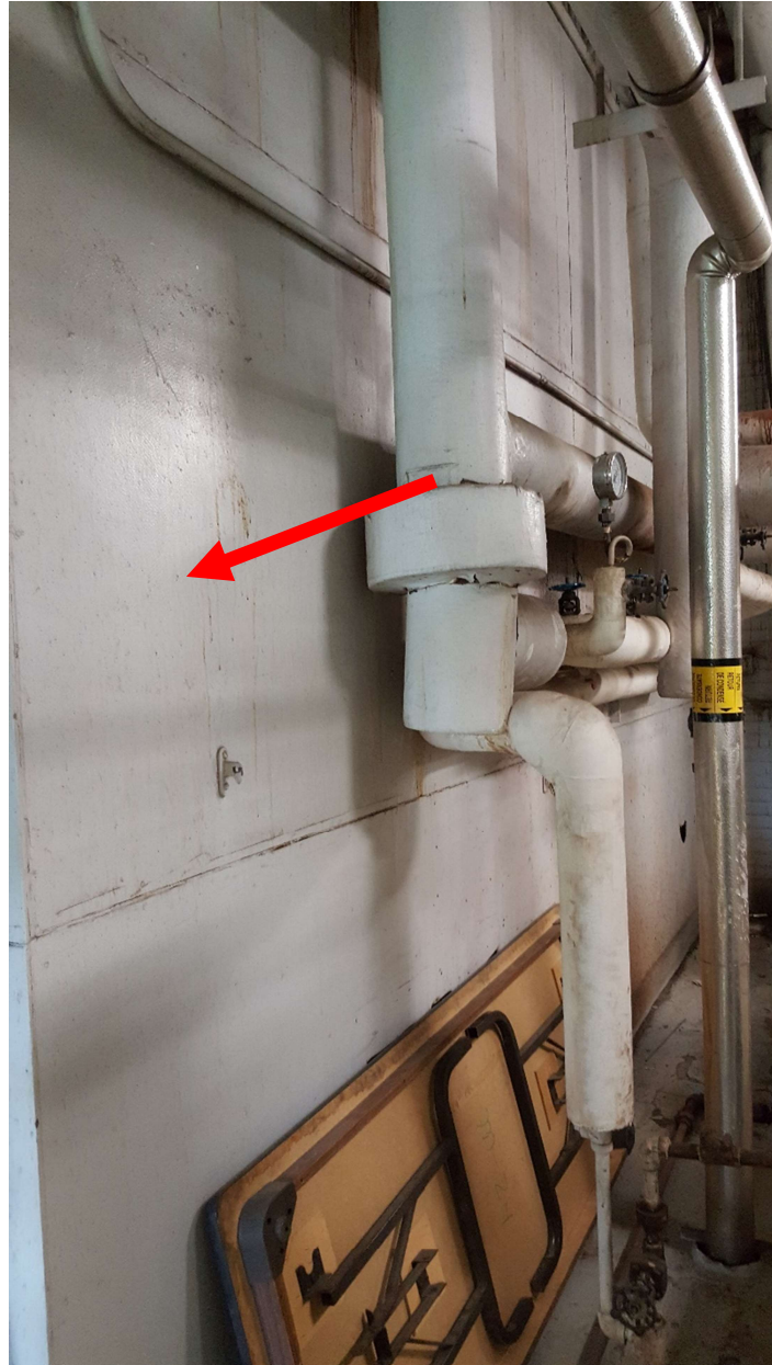
Photograph 2: Asbestos-containing friable fibre board located on the walls of Room 207.
