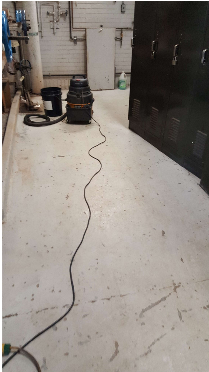
Photograph 8: Lead containing grey paint located on concrete floors throughout the project areas.
