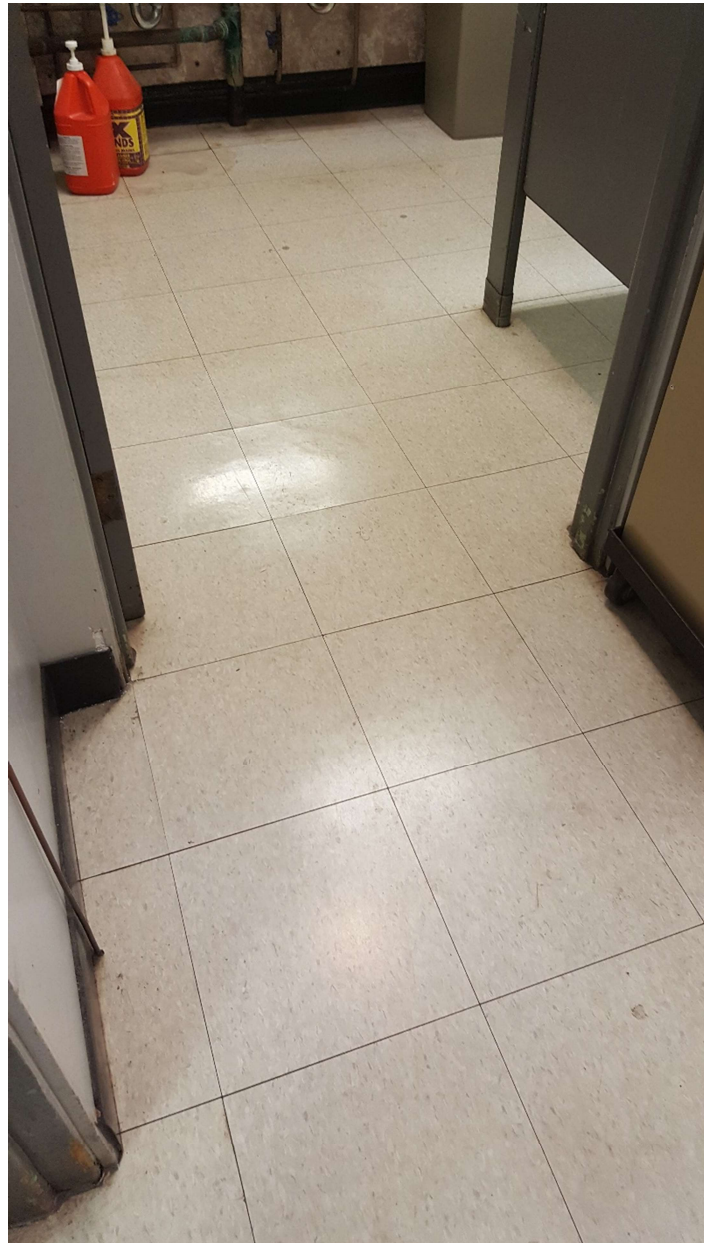
Photograph 1: Asbestos-containing black mastic associated with 12"x12" beige vinyl floor tiles, located in the men's washroom. Since the asbestos-containing mastic cannot be effectively separated from the vinyl tiles, the tiles are also considered asbestos-containing.
