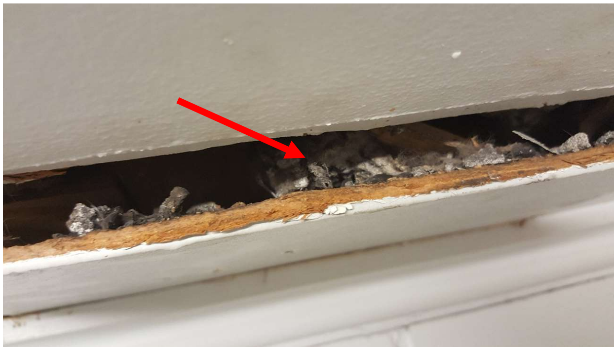
Photograph 4: Asbestos-containing cardboard pipe wrap insulation observed above the ceiling tiles of the men's washroom.
