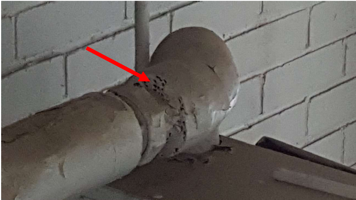
Photograph 5: Asbestos-containing cardboard pipe wrap insulation associated with UNH04/06UNH04 located on the roof above Office 108
