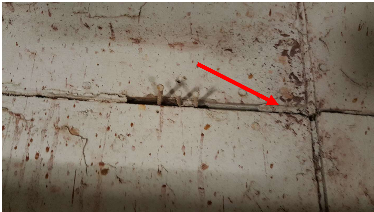
Photograph 3: Asbestos-containing caulking associated with fibre board located on the walls of Room 207.
