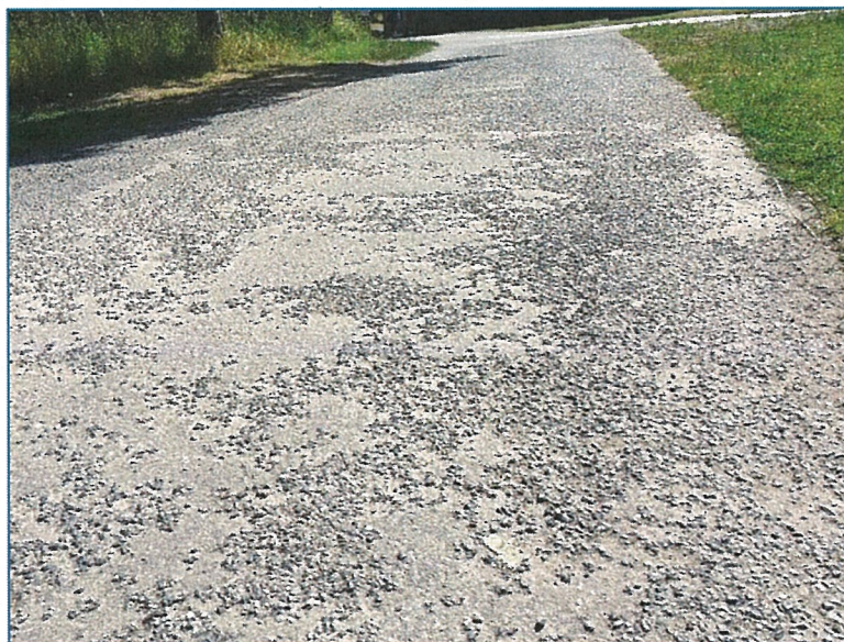
Photo 2 (2017.06.26) – typical surface raveling of the northeast service road
