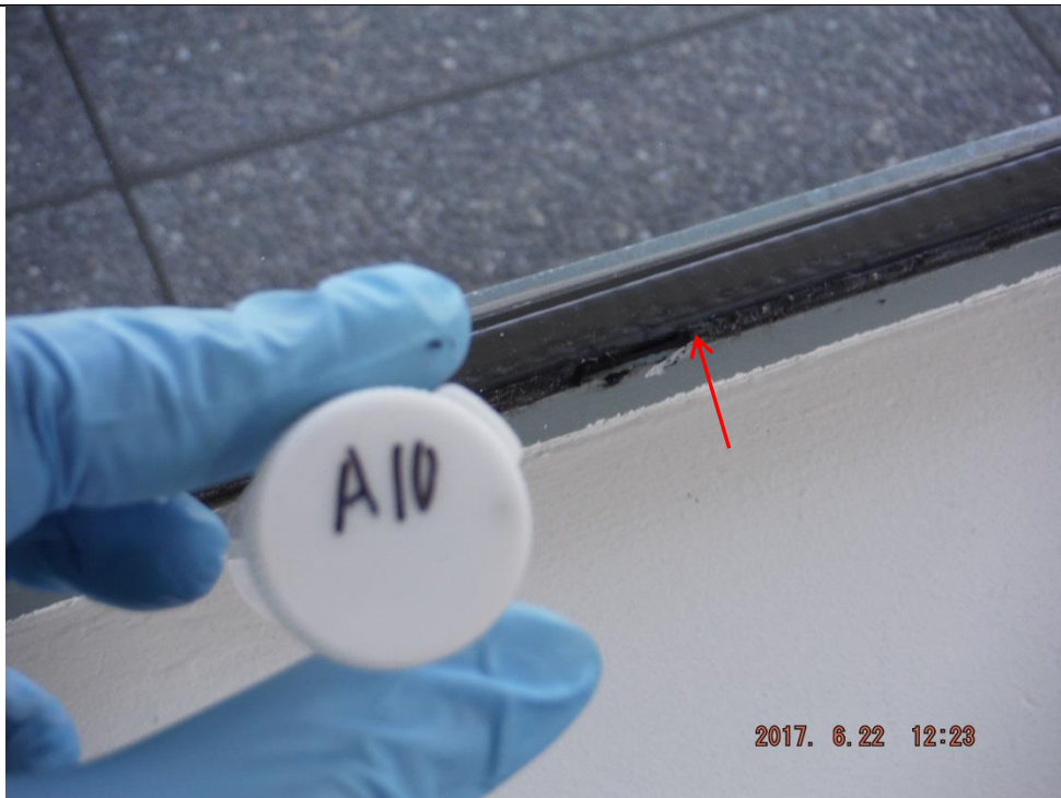
Photo 4 Date: June 21, 2017 Location: 2 nd Floor- Living Room Description: Asbestos-containing black mastic
