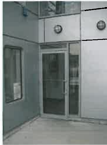
Figure 2.2.1.2 – Storefront glazing: no perimeter sealant; no end dams on head or sill flashings
