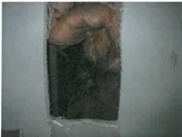
Figure 2.1.9 – Mould and deteriorated exterior sheathing at exploratory opening no: 8
