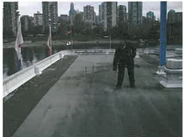
Figure 2.4.5 – Air blister in membrane approx 12" wide
