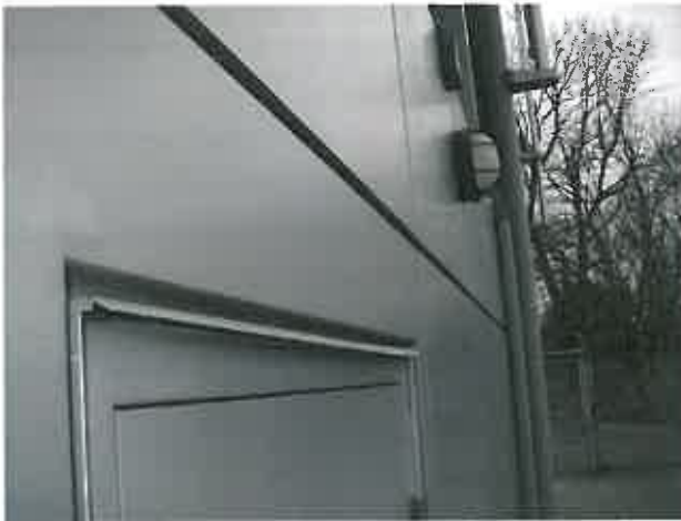
Figure 2.2.2.3 – Head flashings lack end dams
