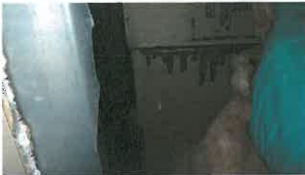
Figure 6 – Brown staining at interior face of exterior sheathing at exploratory opening No. 12.
