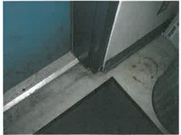
Figure 2.2.2.6 – Corrosion of steel door frame at the interior, near the floor
