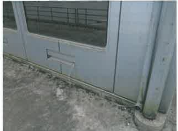
Figure 8 – Typical passive wall vent penetration of exterior wall.
