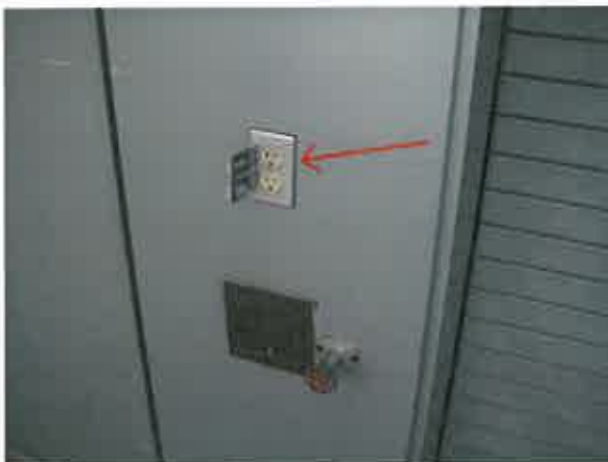
Figure 2.1.7 – Sealant missing at electrical penetration
