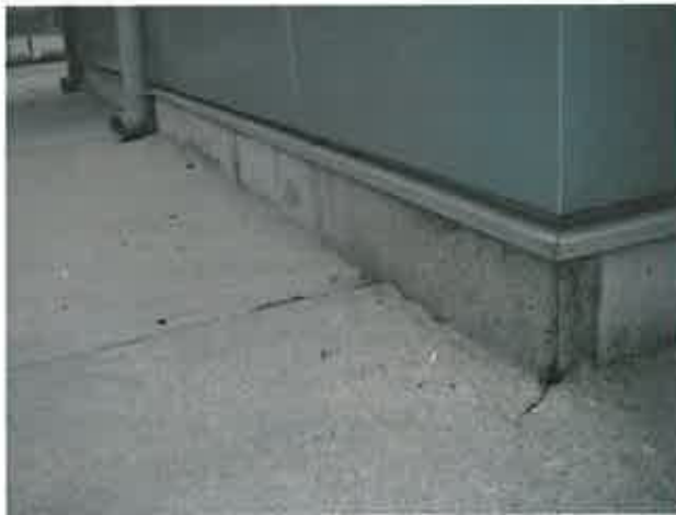
Figure 2.5.1 – Base of wall flashing has little or no slope; joints are lapped and not sealed
