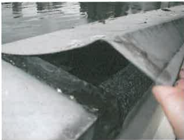
Figure 2.4.3 – Cap flashing lap joints have deteriorated or
