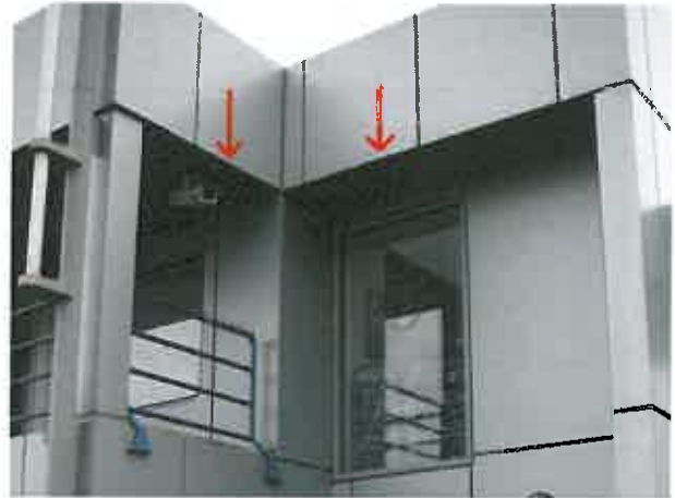
Figure 2.1.2 – No drip flashings provided at base of panels at interface with soffits
