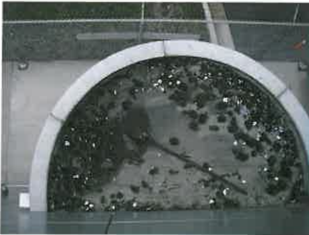
Figure 2.4.8 – Cap flashing of lower secondary roof has lap joints; sealant at joints is missing or deteriorated
