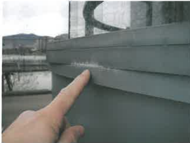
Figure 2.2.1.4 – Minor corrosion between frameless glazing sill and aluminum fascia panel; no sealant installed at this interface
