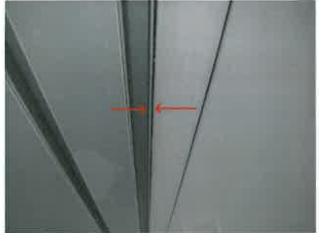
Figure 2.2.2.4 – No perimeter sealant between steel door frame and adjacent cladding
