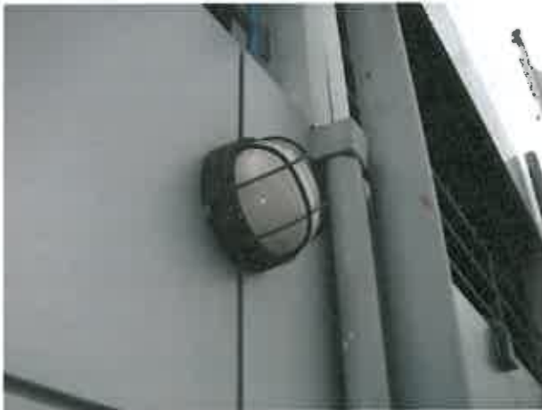
Figure 2.1.6 – Light fixture without perimeter sealant
