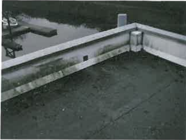
Figure 2.4.7 – Overflow scupper is backsloped towards roof; roof membrane exposed edge terminates inside scupper
