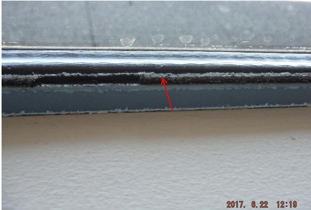
Photo 3 Date: June 21, 2017 Location: 2 nd Floor- Cabin 1 Window Description: Close up photo of asbestos-containing black mastic
