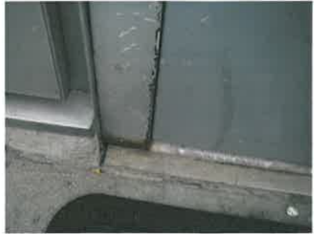
Figure 2.2.2.5 – Corrosion of steel door frame near grade
