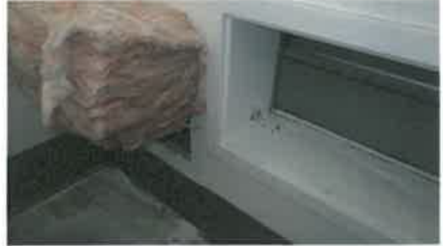
Figure 7 – Deterioration at wood liner at passive wall vent, north elevation, Room 205, D.I.C.
