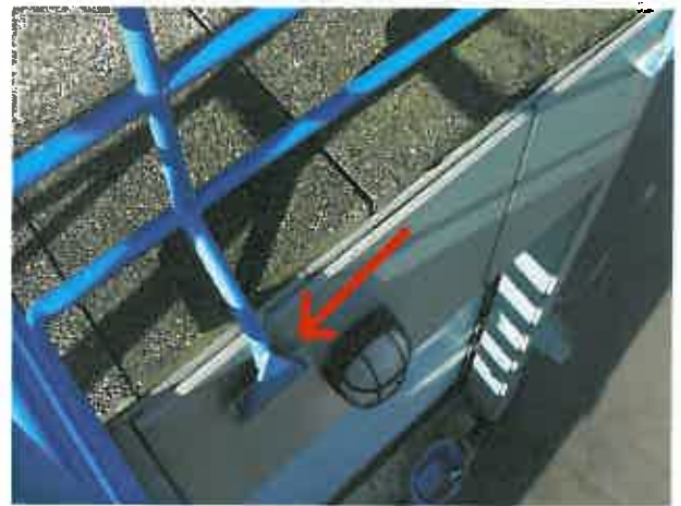
Figure 2.1.4 – Guardrail support penetration with discontinuous sealant at interface with cladding
