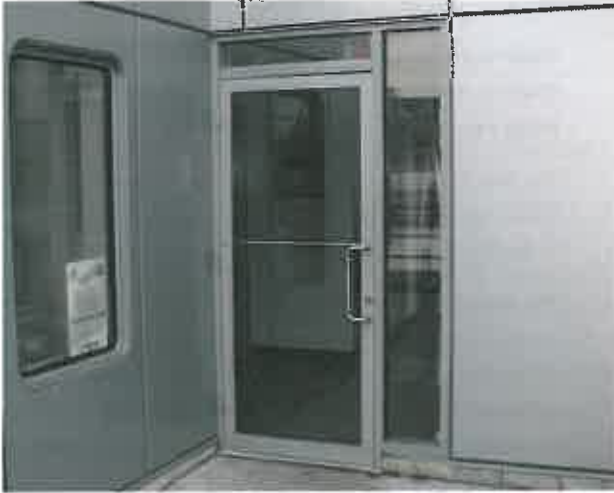
Figure 2.2.2.1 – Storefront swing door has no head flashing
