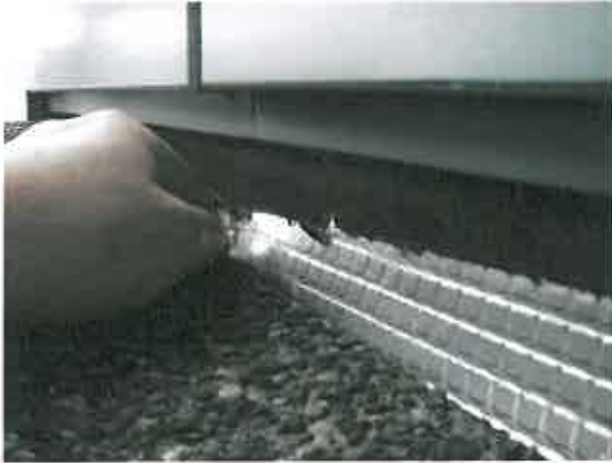
Figure 2.3.1 – Deck membrane is not overlapped by cladding or wall membrane above
