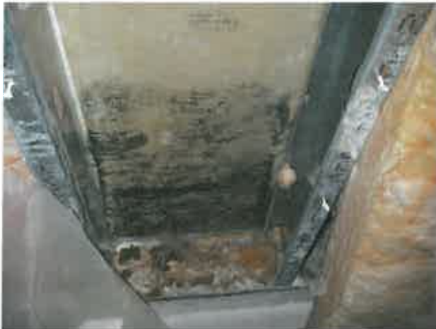
Figure 2.1.8 – Mould and deteriorated exterior sheathing at exploratory opening no: 1G
