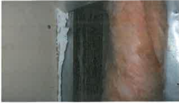
Figure 4 – Exploratory opening No. 12. Corrosion on structural steel column within exterior wall assembly.
