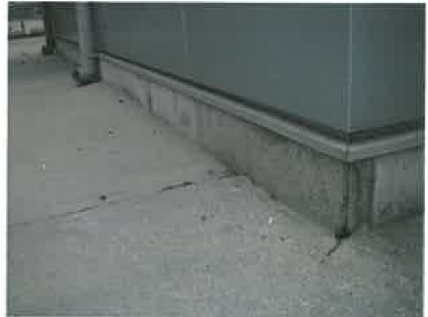
Figure 2.1.3 – Base flashing of wall has little or no slope and horizontal lap joints
