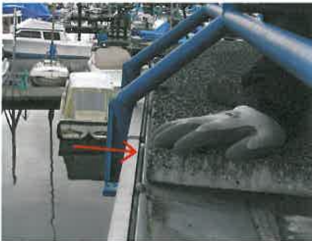
Figure 2.1.1 – Deteriorated perimeter gaskets at aluminum cladding panels
