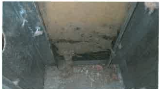
Figure 2 – Exploratory opening No. 8. Mould on interior face of paper-faced exterior gypsum board sheathing.
