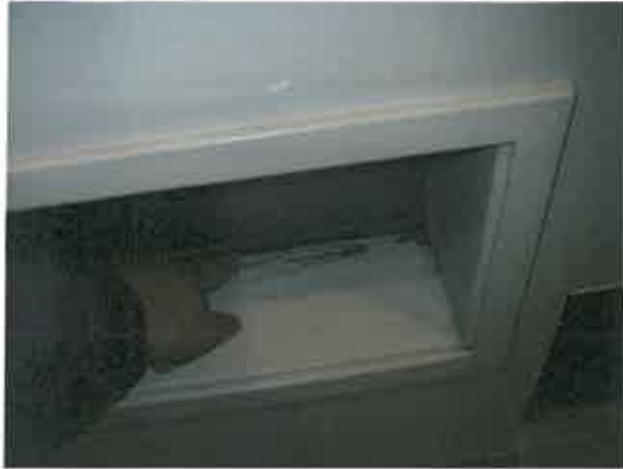
Figure 2.6.1 – Deteriorated wood trim at fresh air vent
