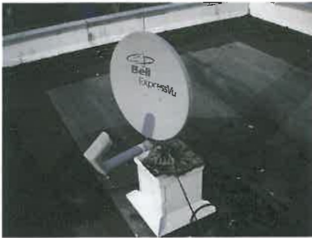
Figure 2.4.1 – Receiver dish installed on roof pedestal
