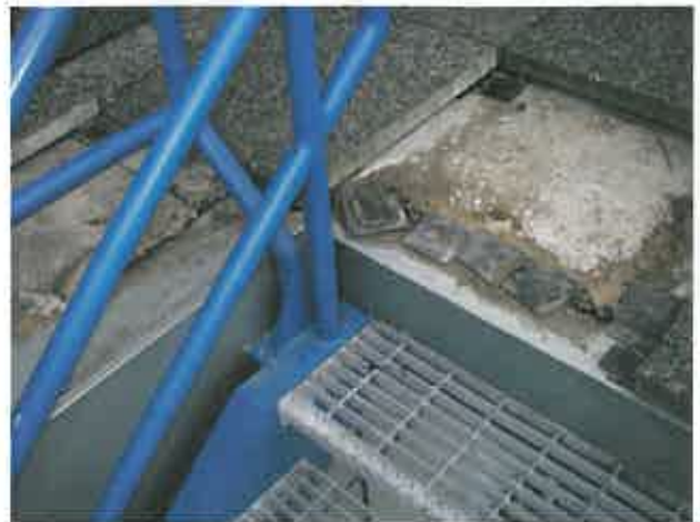
Figure 2.3.4 – Granular substance on membrane at location of past repair
