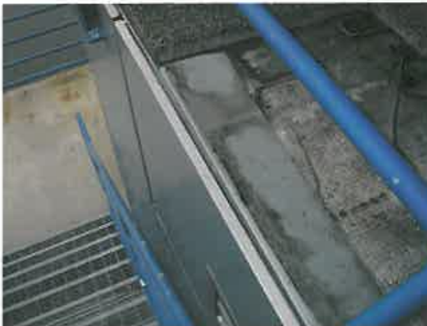
Figure 2.3.2 – Flashing at outboard edge of deck has lap joints and no sealant at the joints
