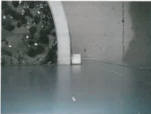
Figure 2.4.9 – Sealant at scupper box to cladding interface is deteriorated; sealant at cap flashing to cladding interface is deteriorated
