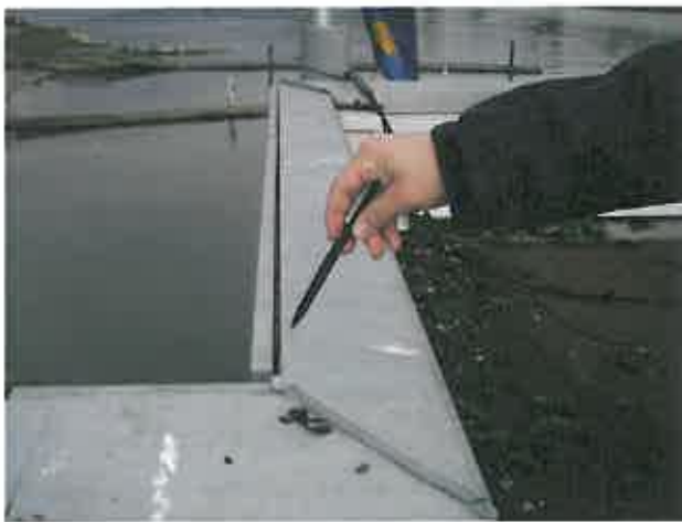
Figure 2.4.2 – Cap flashing does not overlap wall cladding
