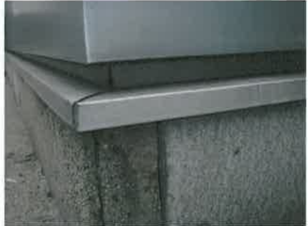
Figure 2.5.2 – Cement board joints are open adjacent to grade
