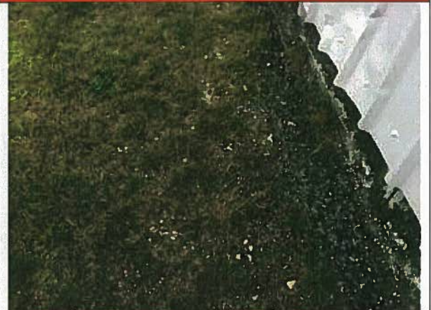
Sample: 27384-6 Location: West Exterior of the Building Description: Mastic Debris Hazardous Material: Chrysotile 8%
