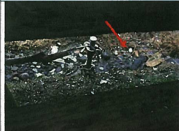
Sample: 27384-5 Location: West Exterior of the Building Description: Mastic Debris Hazardous Material: Chrysotile 8%
