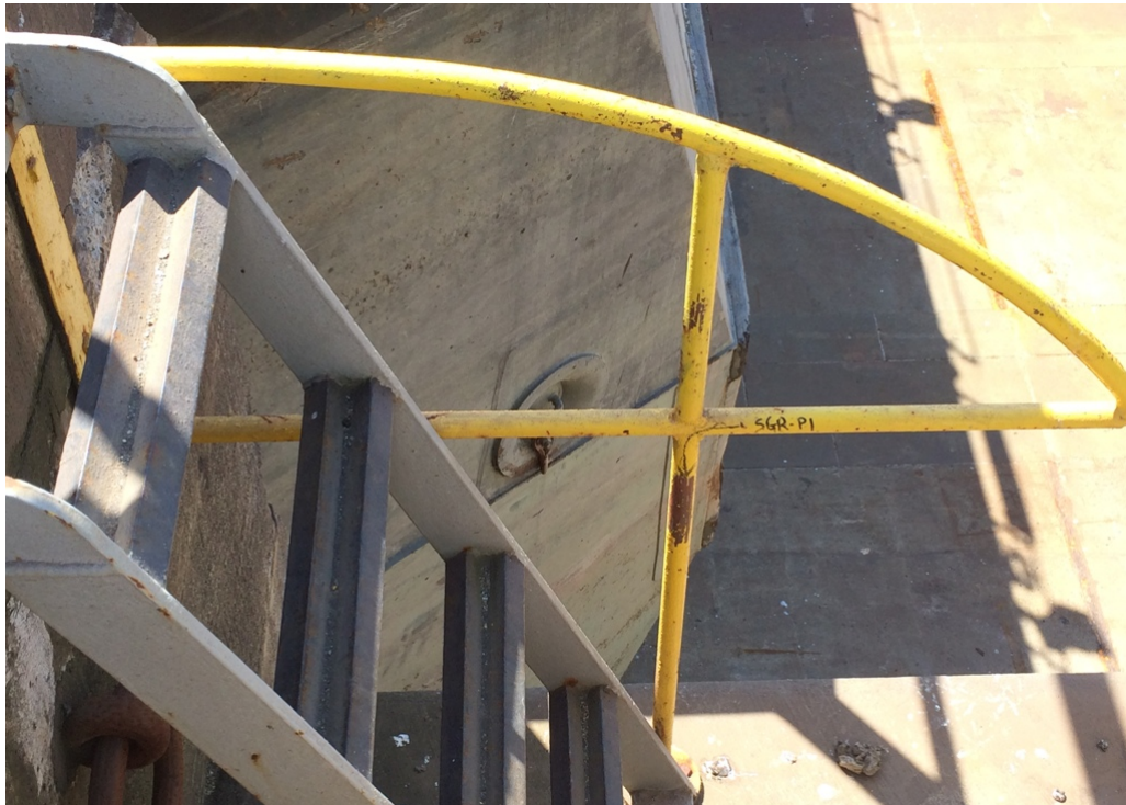
Photograph 7: Lead-based yellow paint on the sill guard railing on the north side of the west graving dock. Sample SGR-P1. Sample SGR-P2, P3, and P8 similar (photo not provided).
