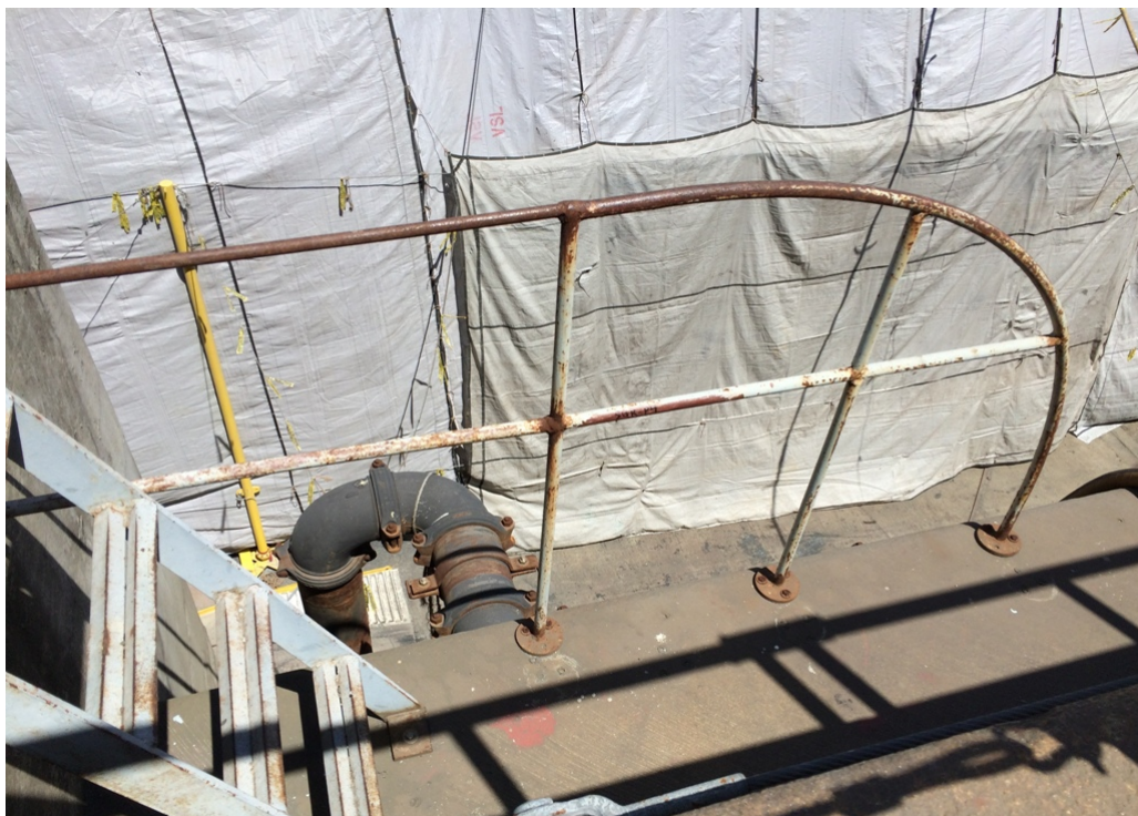
Photograph 8: Lead-based grey paint on the sill guard rail on the south side of the east graving dock. Sample SGR-P4. Sample SGR-P5, P6, and P7 similar (photo not provided).
