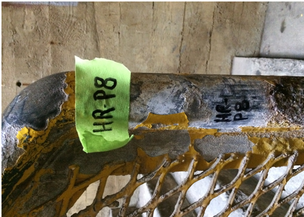
Photograph 6: Lead based yellow paint on the hand rail at the lower landing of the dock bottom middle stairwell. Sample HR-P8
