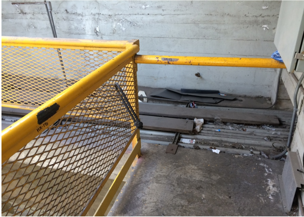
Photograph 5: Lead-based yellow paint on the hand and guard rails in the dock bottom middle stairwell. Samples HR-P6 and HR-P7.
