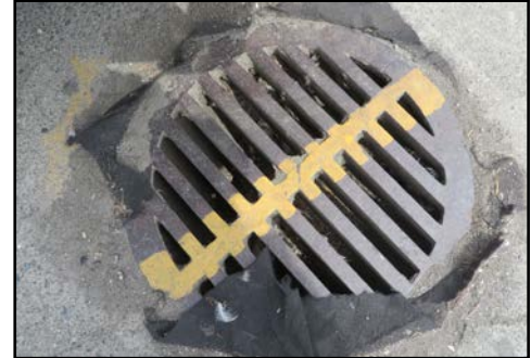
Uplands storm drain with filter cloth. Avoid storing hazardous materials near storm drains, which are directly linked to the marine environment.
