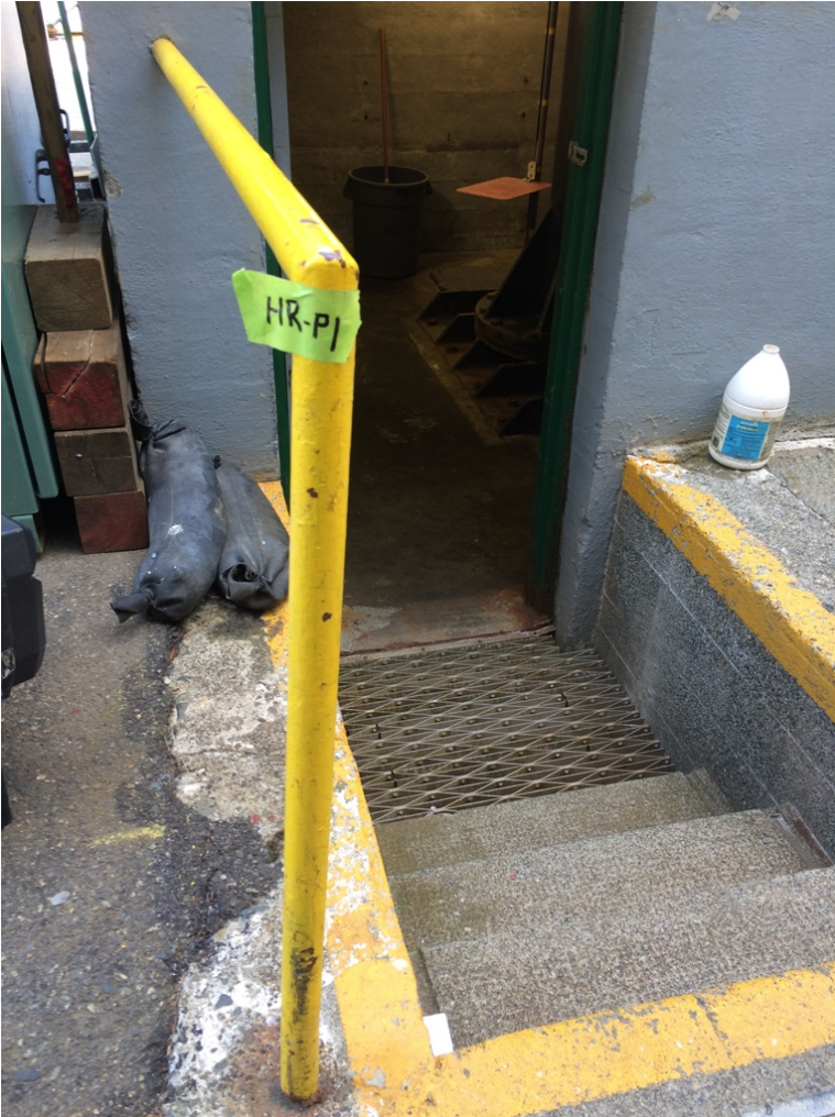
Photograph 1: Lead-based yellow paint on the main Penstock Building entrance hand railing. Sample HR-P1.
