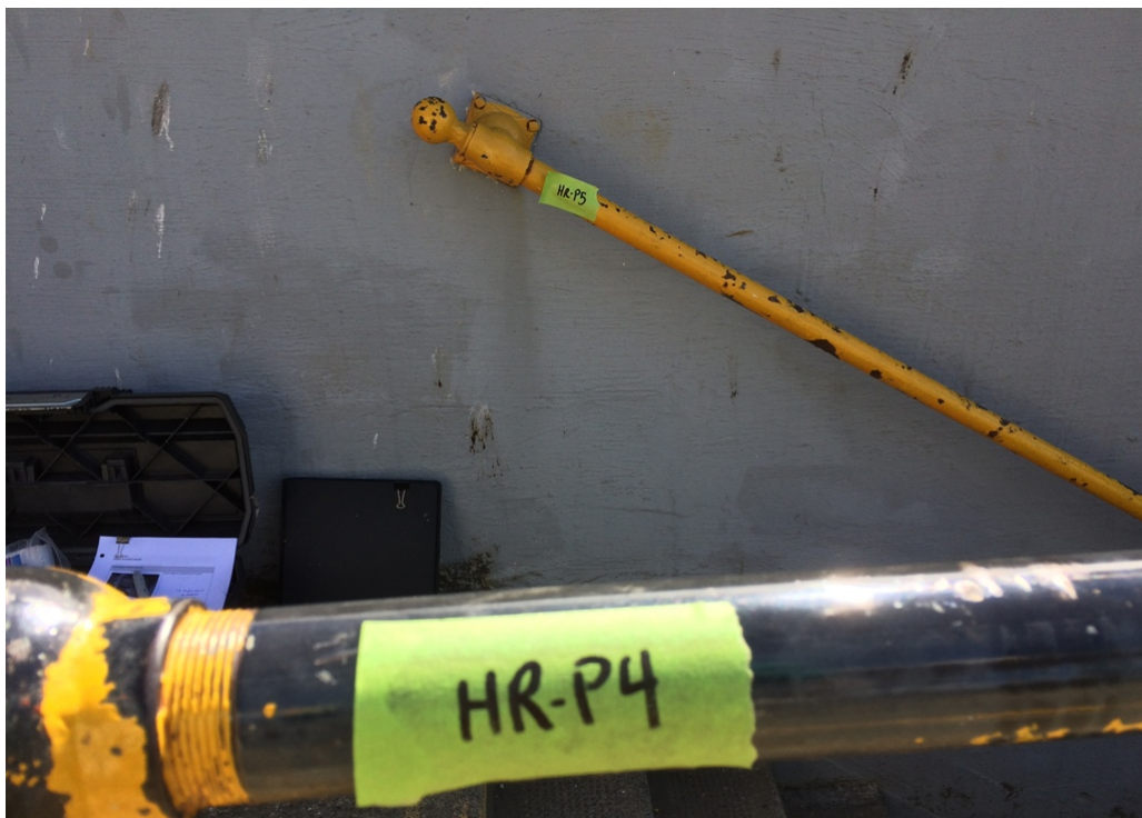
Photograph 4: Lead-based yellow paint on the hand and guard rails at the dock bottom middle stairwell entrance. Samples HR-P4 and HR-P5.
