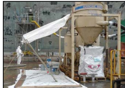
All hazardous materials must be stored in appropriate containment and away from tunnel drain system.
