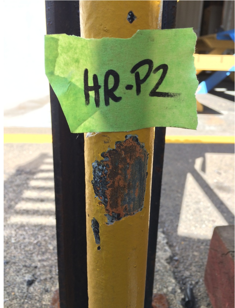
Photograph 2: Lead-based yellow paint on the west entrance hand railing to the middle Penstock Building. Sample HR-P2.
