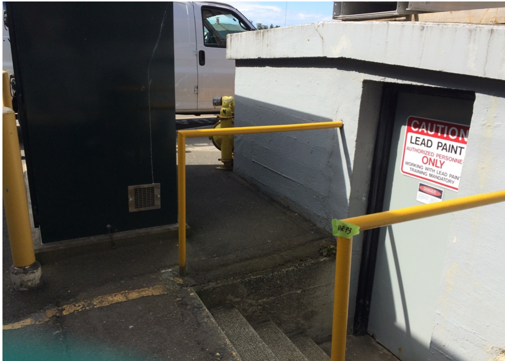
Photograph 3: Lead-based yellow paint on the east entrance hand railing to the middle Penstock Building. Sample HR-P3.
