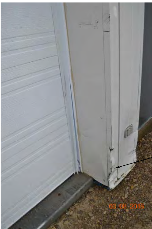
1 DETAIL 2 - DAMAGED GARAGE DOOR A2.3 SCALE: NTS
