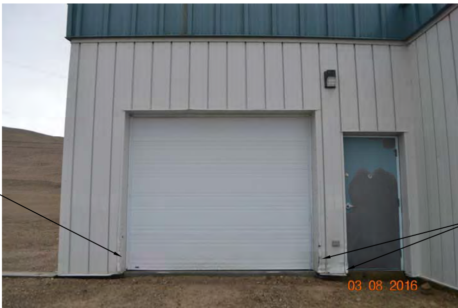
1 DETAIL 1 - DAMAGED GARAGE DOOR A2.3 SCALE: NTS
