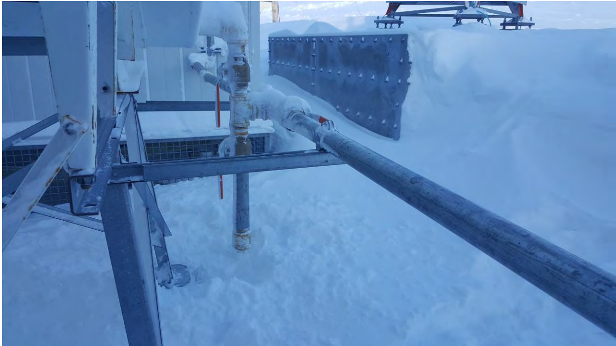
Photo 19 Facility Building Piping
