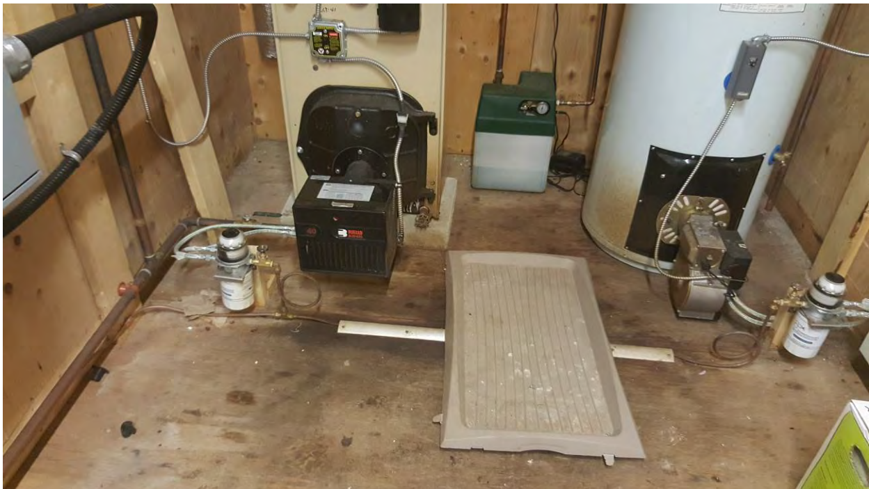
Photo 14 - Typical Interior Piping
