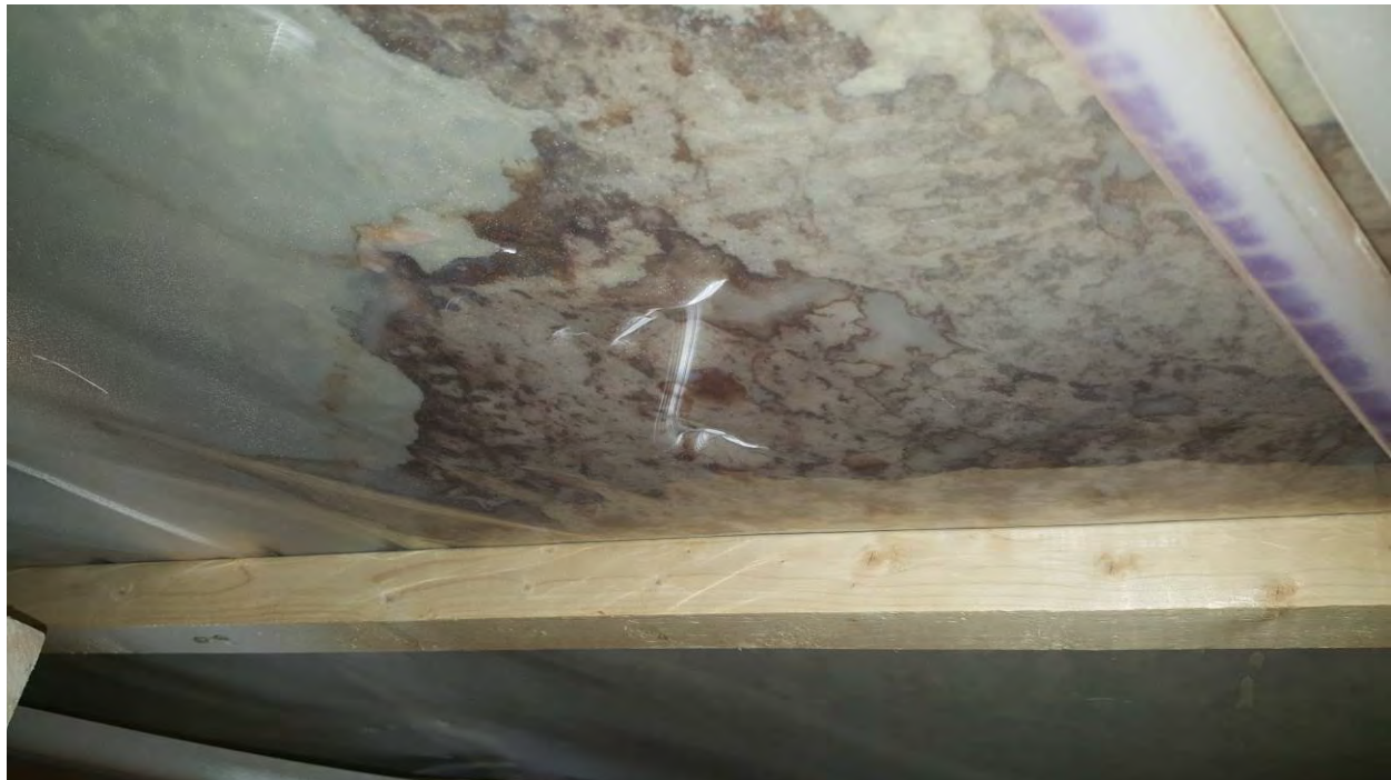
Photo 4 Water Damage at Ceiling
