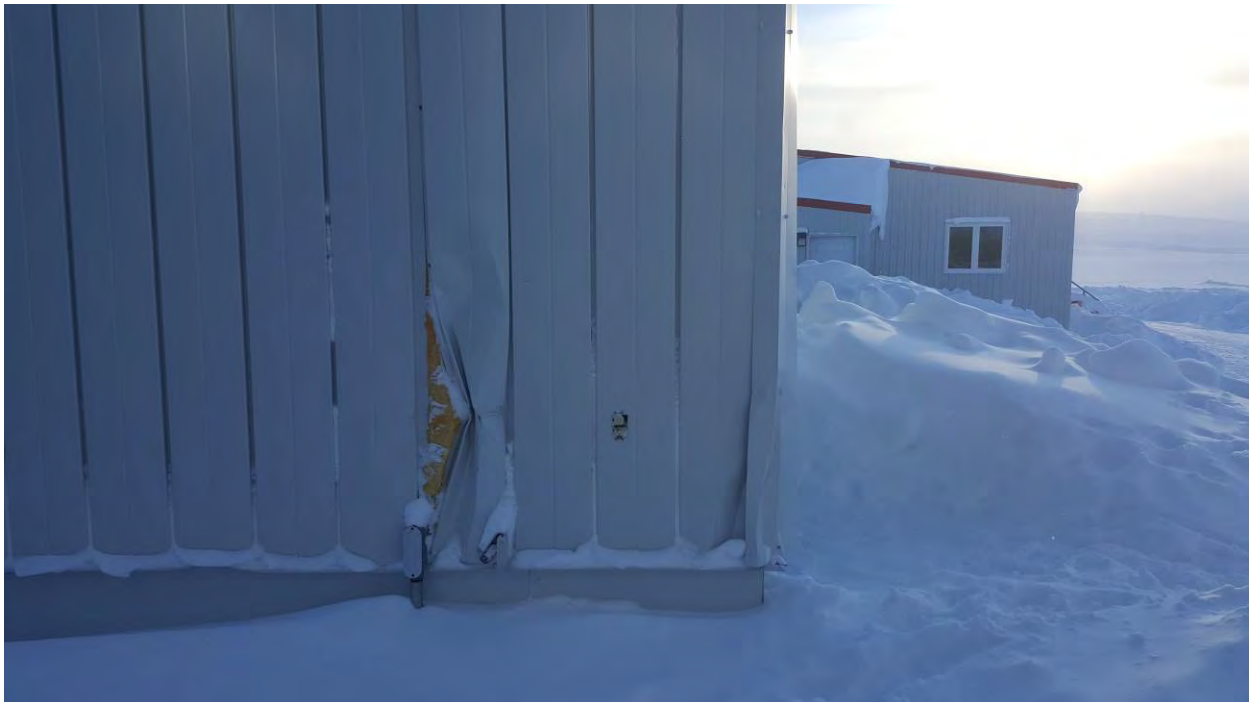
Photo 24 Damage to Garage
