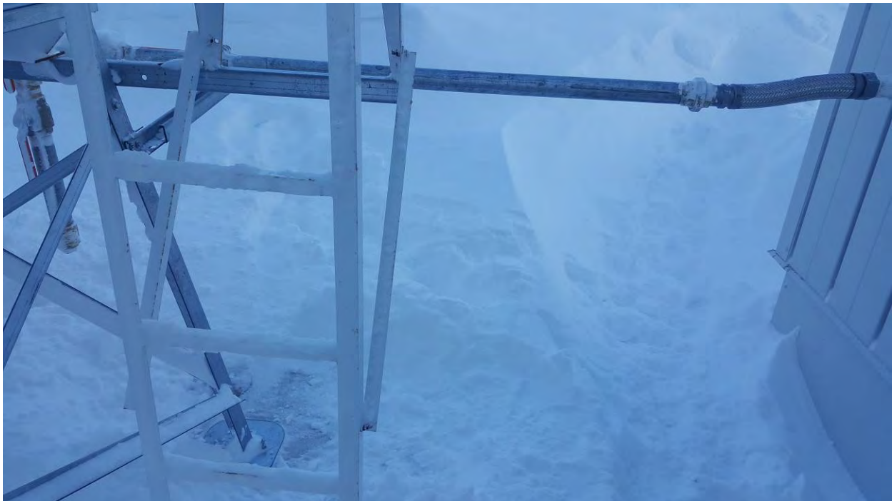
Photo 20 Facility Building Piping
