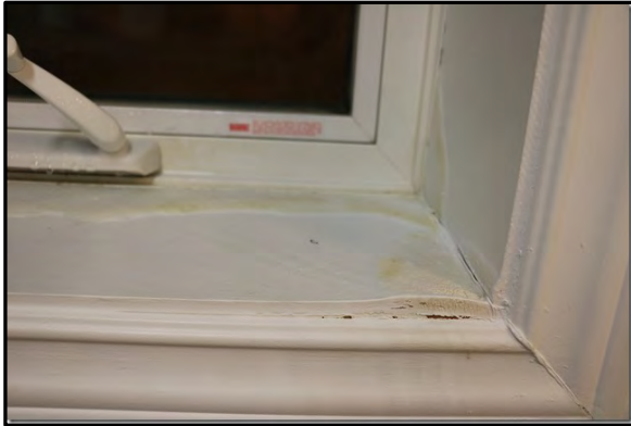
Photo #1 – Water damage on the Bedroom 2 window of Building B prior to assessment.
