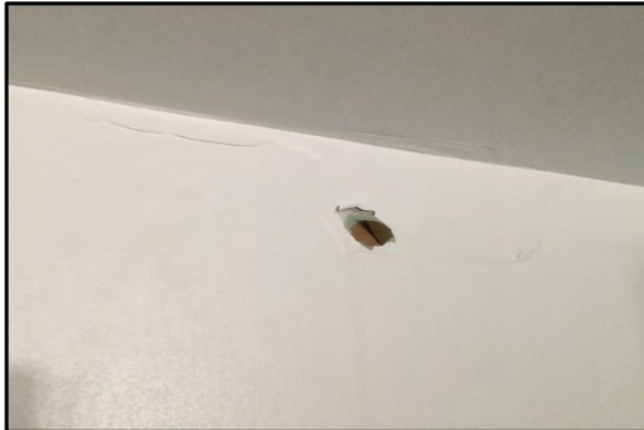
Photo #17 – Bubbled paint and water staining above on the wall above the shower in Building B.
