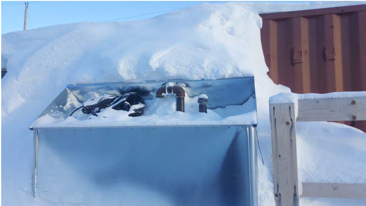
Photo 13 - Existing Oil Tank
