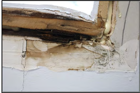
Photo #2 – Mould growth on the Bedroom 2 window sill of Building B prior to assessment.
