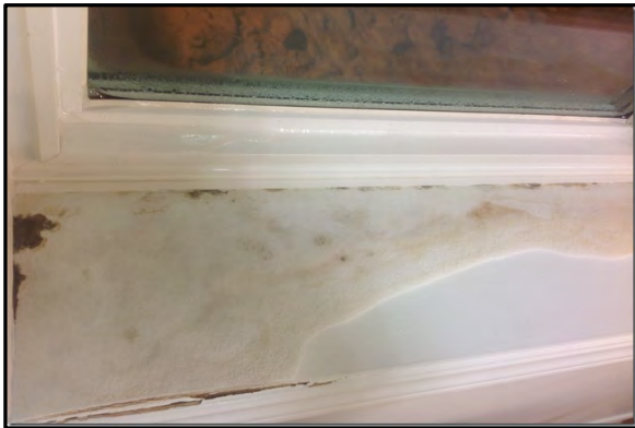
Photo #3 – Water damage on the kitchen window of Building B prior to assessment.
