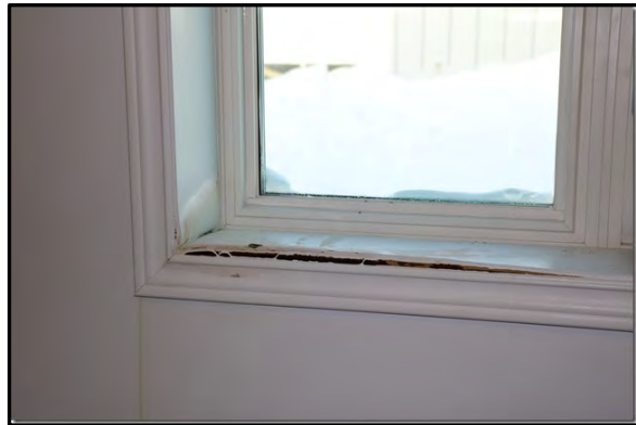
Photo #4 – Water damaged MDF and staining on kitchen wall of Building B prior to assessment.
