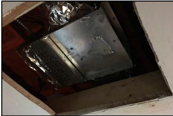
Photo #15 – Ice on the bottom the HRV pre-heater in Building B.
