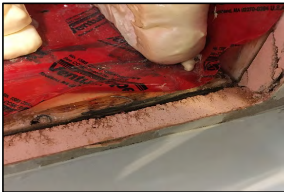
Photo #11 – Water damaged gypsum board, wood at the kitchen window sill of Building A.
