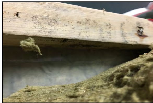
Photo #12 – Mould growth on the wood at the Building A, Bedroom 2 window sill.
