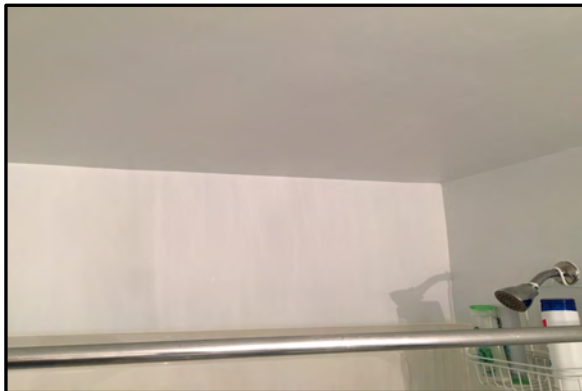
Photo #19 – Water stained paint above the shower in the bathroom above of Building A.
