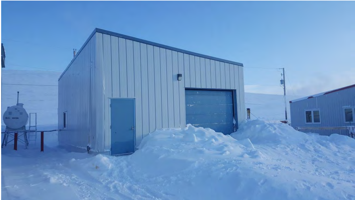
Photo 23 - Damage To Garage
