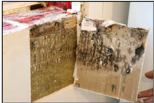
Photo #6 – Mould damaged drywall below kitchen window of Building B prior to assessment.
