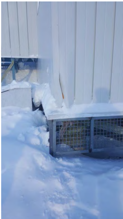
Photo 22 Damage to Facility Building
