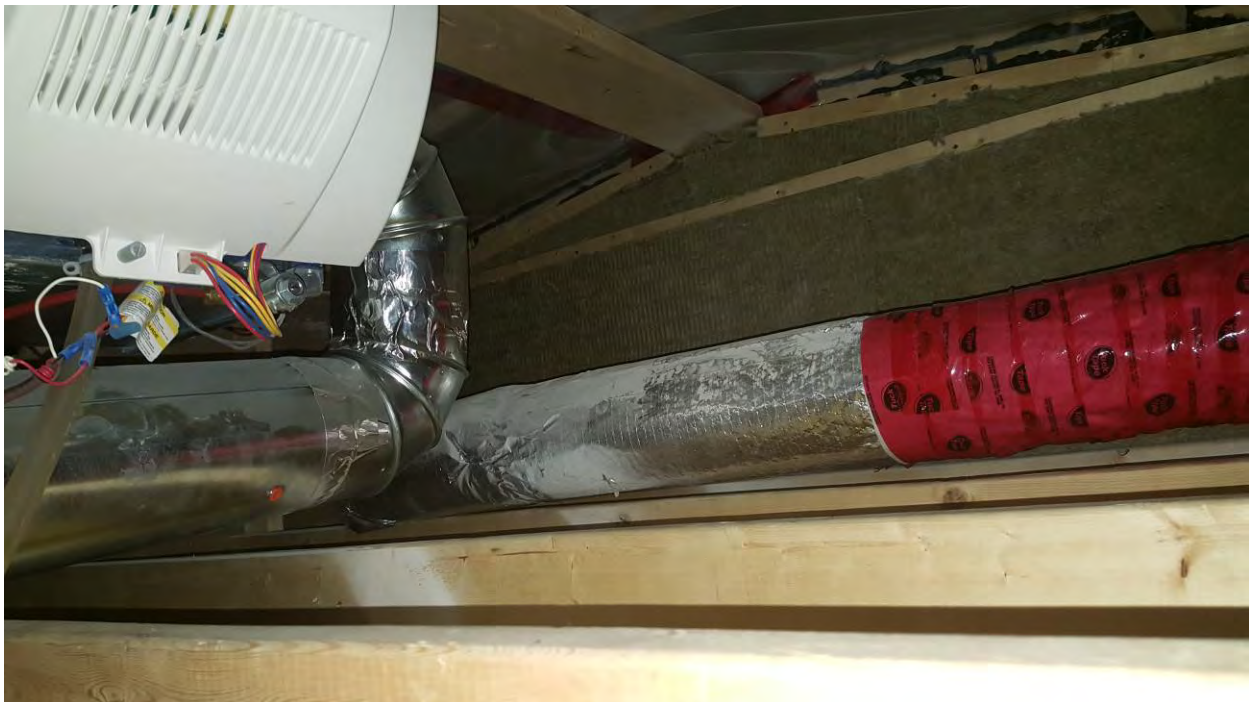
Photo 2 HRV ducts to be insulated
