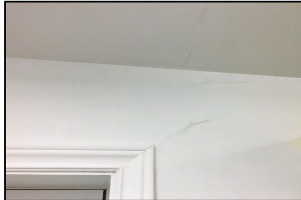
Photo #18 – Cracked gypsum board and bubbled paint above the exterior doorway in the laundry room Building B.
