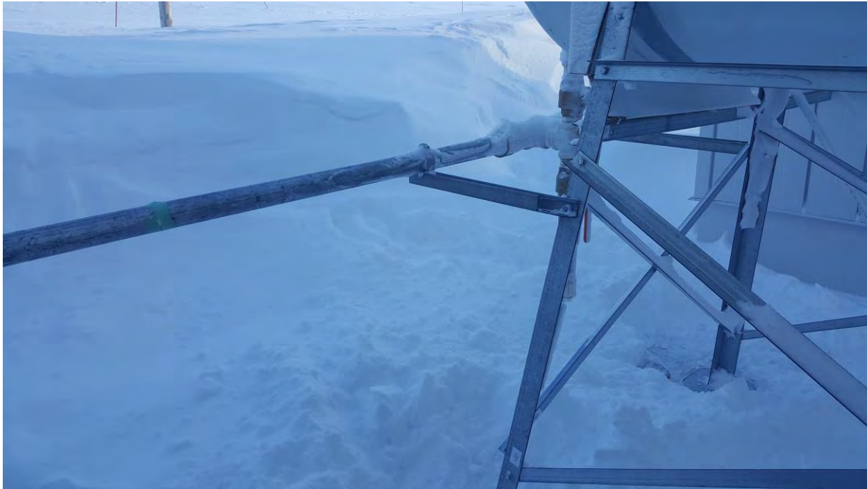
Photo 21 Facility Building Piping
