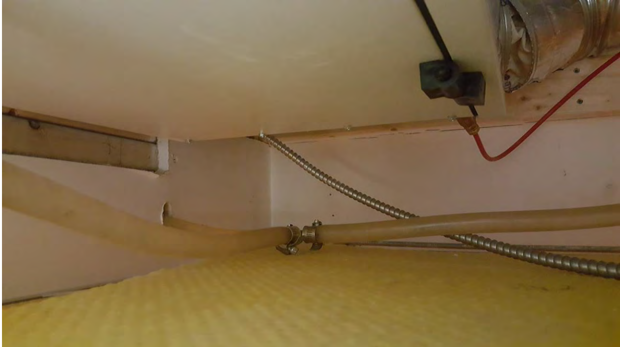
Photo 1- HRV and Humidifier Drain Lines
