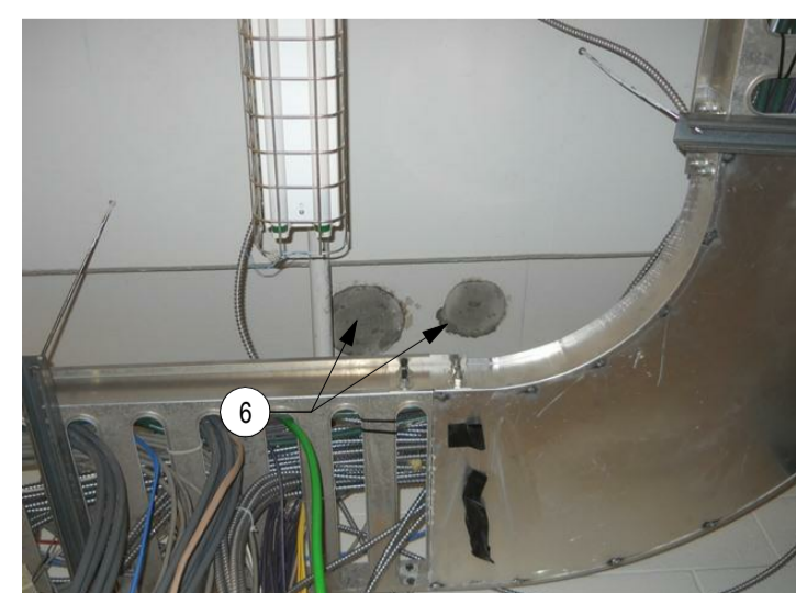
ROOM 006 - SERVER ROOM PHOTO 104
