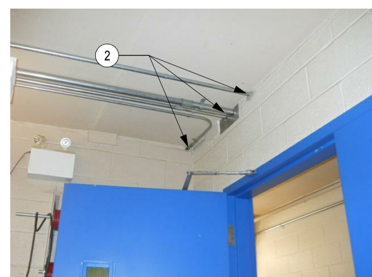
ROOM 012 - ELECTRICAL SHOP PHOTO 138
