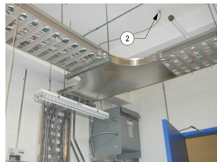
ROOM 006 - SERVER ROOM PHOTO 088
