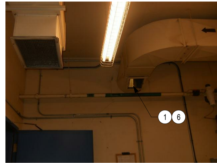
ROOM 013 - COMPRESSOR ROOM PHOTO 148
