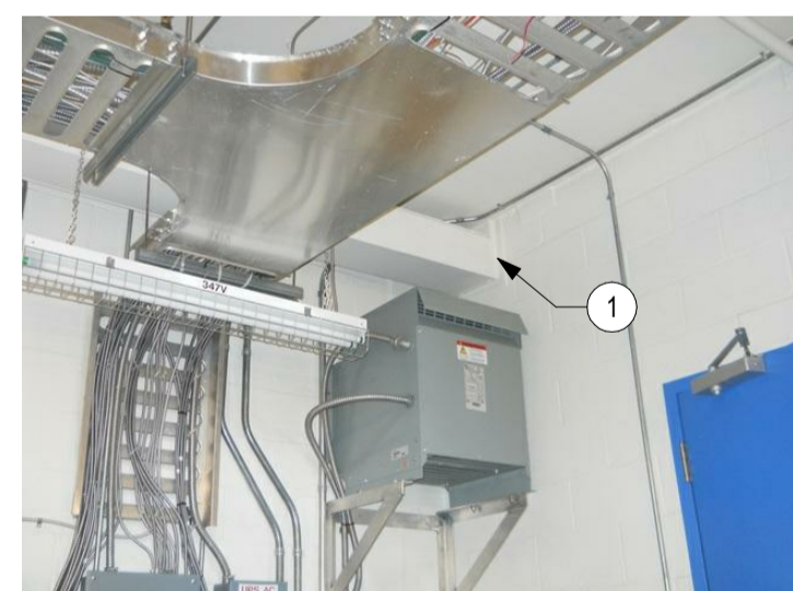
ROOM 006 - SERVER ROOM PHOTO 096
