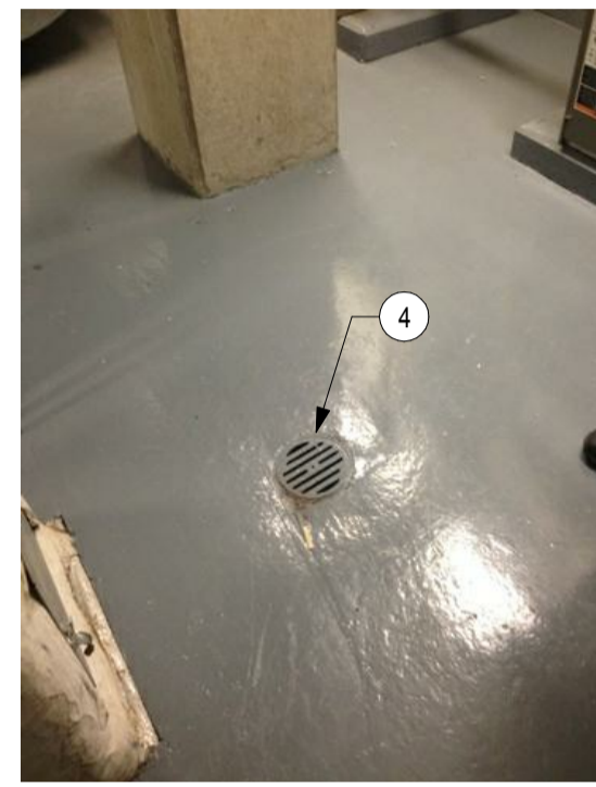
ROOM 211 - MECHANICAL ROOM PHOTO 250
