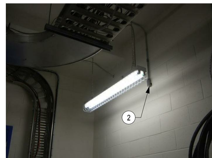
ROOM 006 - SERVER ROOM PHOTO 090
