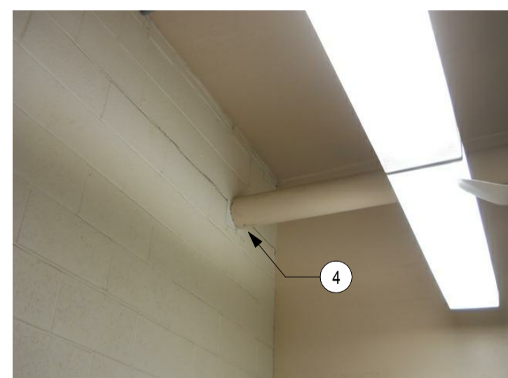
ROOM 012 - ELECTRICAL SHOP PHOTO 130
