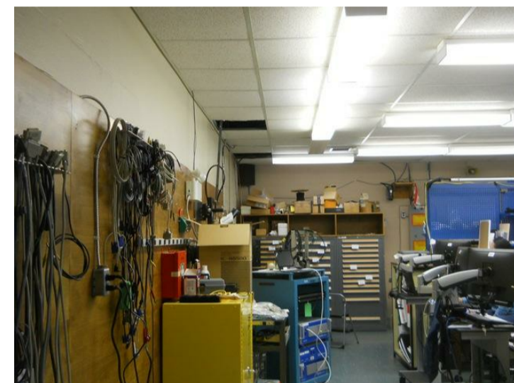
ROOM 010 - T & E WORKSHOP PHOTO 120
