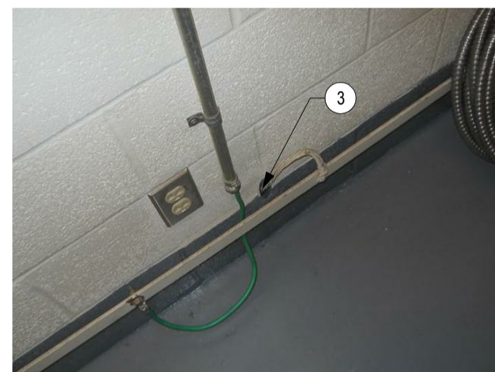
ROOM 015 - ELECTRICAL ROOM PHOTO 160
