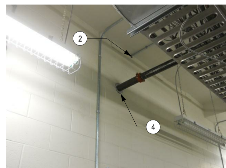
ROOM 006 - SERVER ROOM PHOTO 098
