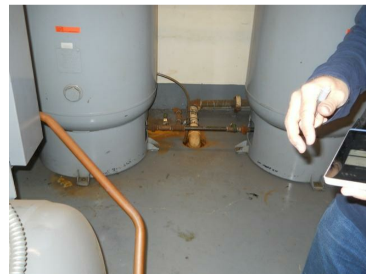
ROOM 013 - COMPRESSOR ROOM PHOTO 154
