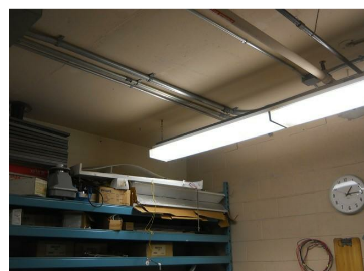
ROOM 012 - ELECTRICAL SHOP PHOTO 136
