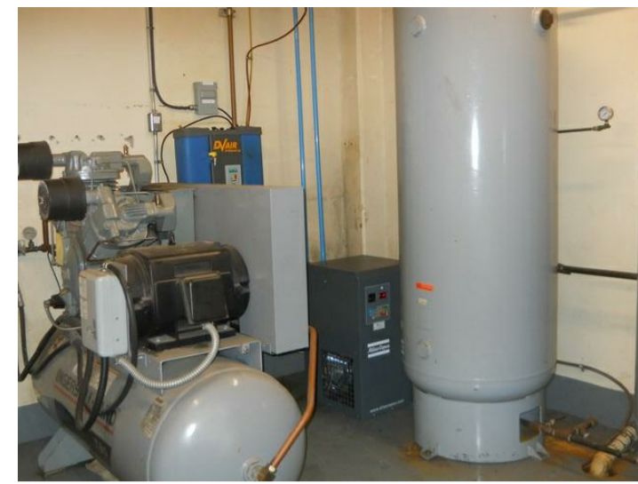
ROOM 013 - COMPRESSOR ROOM PHOTO 146
