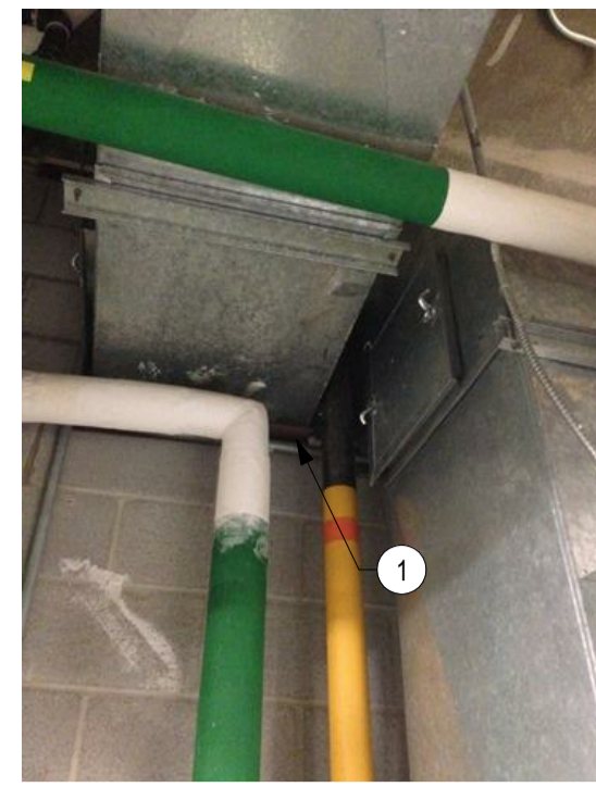
ROOM 211 - MECHANICAL ROOM PHOTO 247
