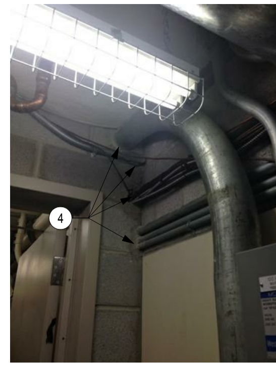
ROOM 211 - MECHANICAL ROOM PHOTO 246
