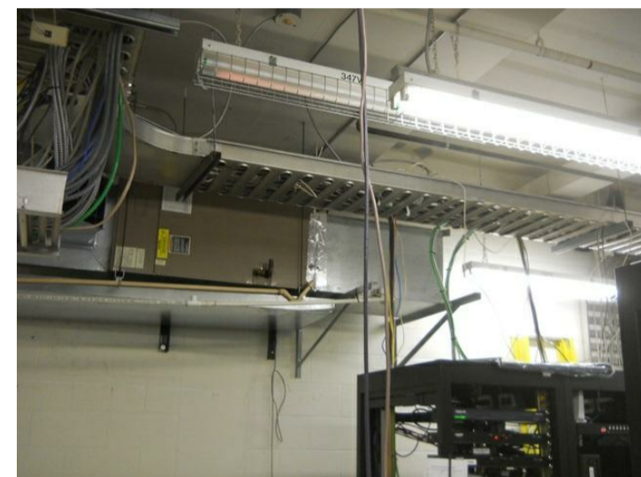
ROOM 006 - SERVER ROOM PHOTO 083
