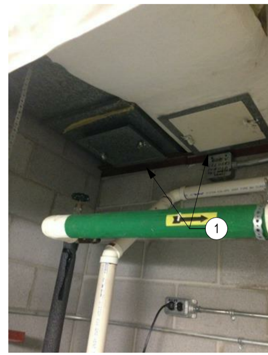
ROOM 211 - MECHANICAL ROOM PHOTO 248
