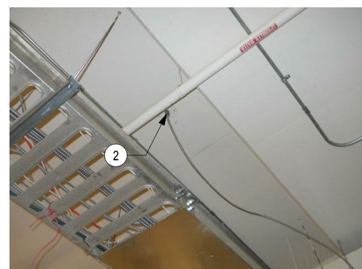
ROOM 006 - SERVER ROOM PHOTO 095
