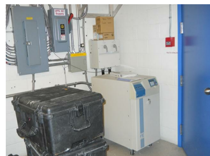
ROOM 006 - SERVER ROOM PHOTO 097
