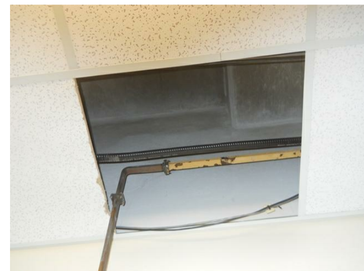
ROOM 010 - T & E WORKSHOP PHOTO 121
