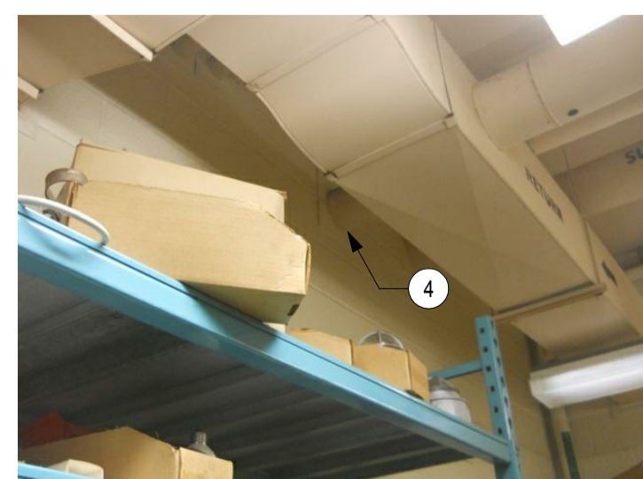
ROOM 012 - ELECTRICAL SHOP PHOTO 140
