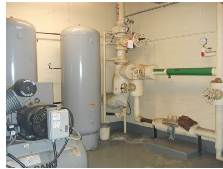
ROOM 013 - COMPRESSOR ROOM PHOTO 145
