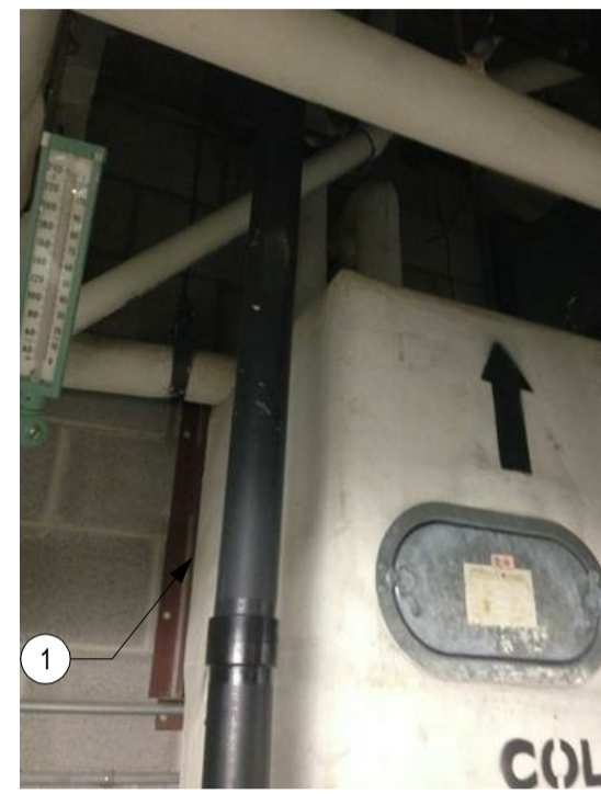
ROOM 211 - MECHANICAL ROOM PHOTO 249
