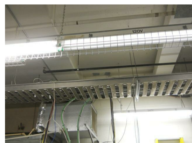
ROOM 006 - SERVER ROOM PHOTO 101
