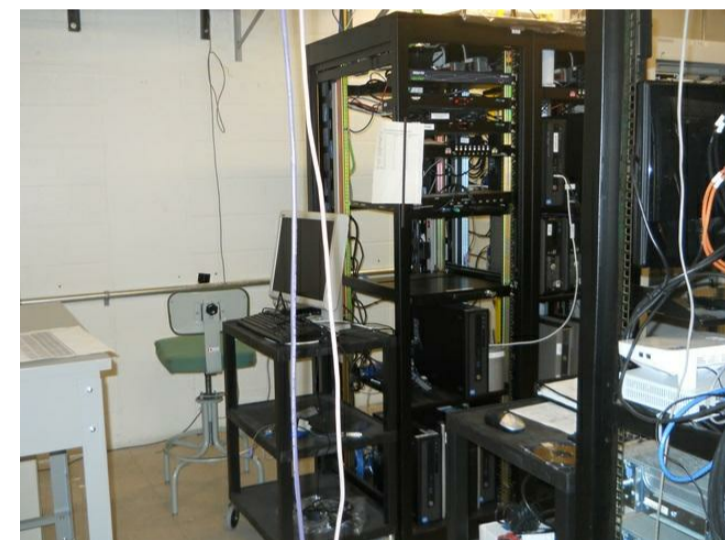
ROOM 006 - SERVER ROOM PHOTO 084
