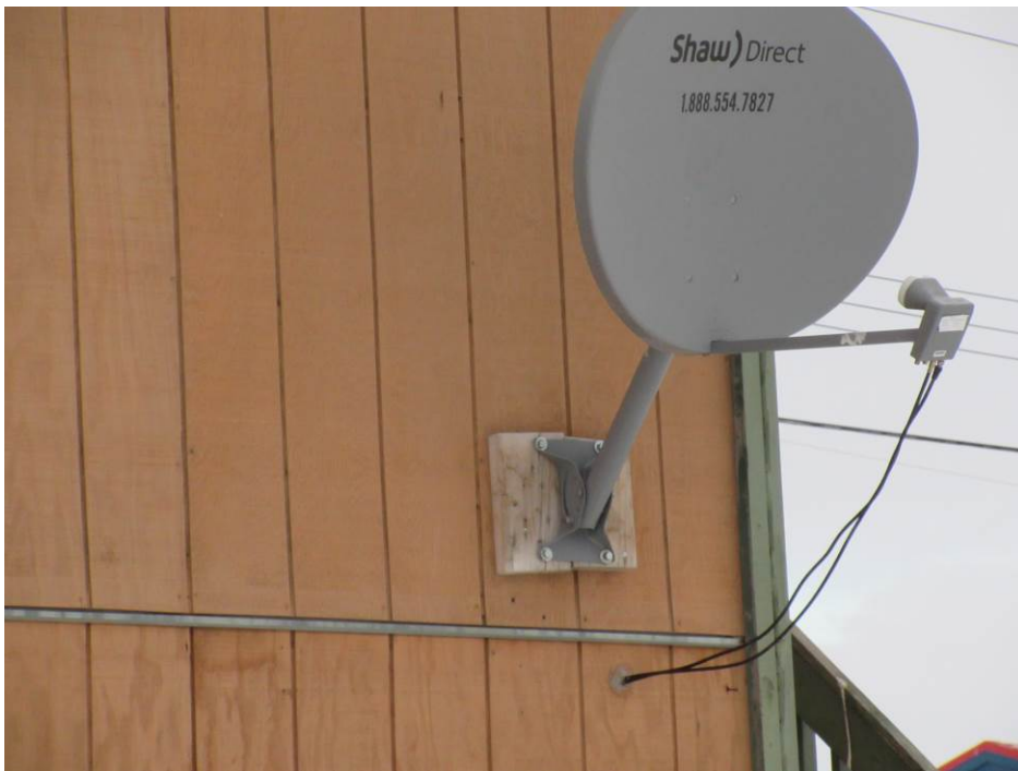
Photo 14 Existing Satellite Dish
