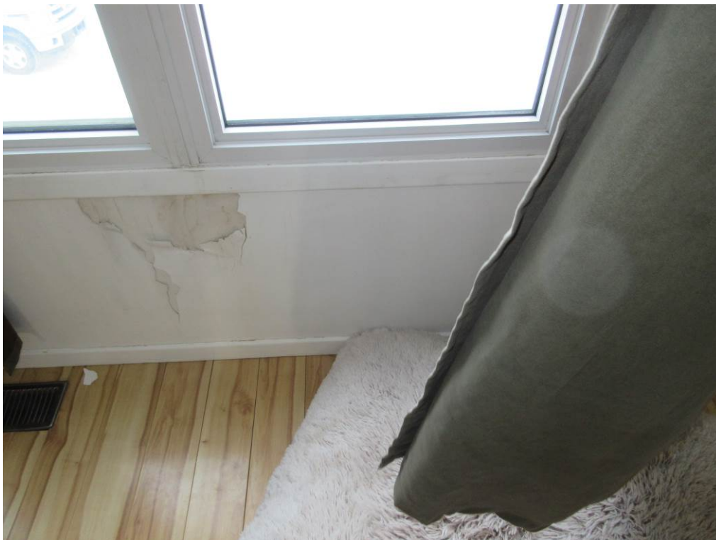
Photo 12 Damaged Front Window
