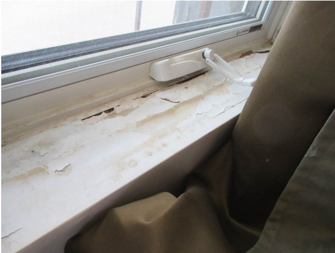
Photo 11 Damaged Dining Room Window
