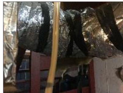
Photograph No. 3 – All piping in both building are either uninsulated, or insulated with fibreglass.
