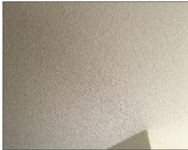
Photograph No. 1 – Texture coat on the drywall ceilings in the Souris residence.
