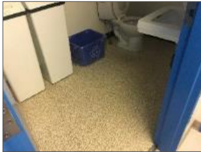
Photograph No. 8 – Asbestos-containing tan vinyl sheet flooring present in the Souris detachment.
