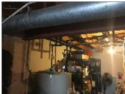
Photograph No. 2 – All piping in both building are either uninsulated, or insulated with fibreglass.
