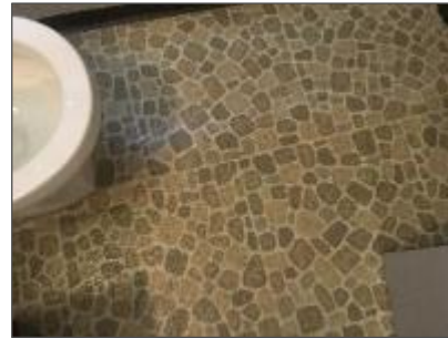
Photograph No. 9 –Asbestos containing vinyl sheet flooring in the 2 nd floor bathroom of the Minnedosa detachment.
