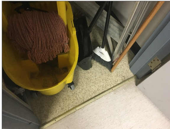
Photograph No. 11 – Vinyl sheet flooring from the main floor janitors closet in the Minnedosa detachment.
