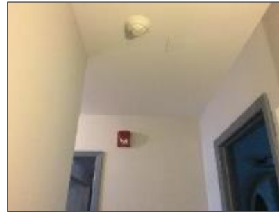
Photograph No. 7 – Drywall as a wall and ceiling finish in the Minnedosa detachment.
