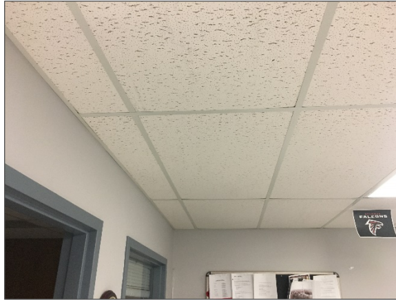
Photograph No. 10 – 24” x 48” acoustic ceiling tiles sampled from the main floor of the Minnedosa detachment (samples 0012A-C).
