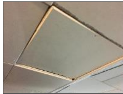
Photograph No. 5 – 12" x 12" ceiling tiles sampled from the basement of the Souris residence.
