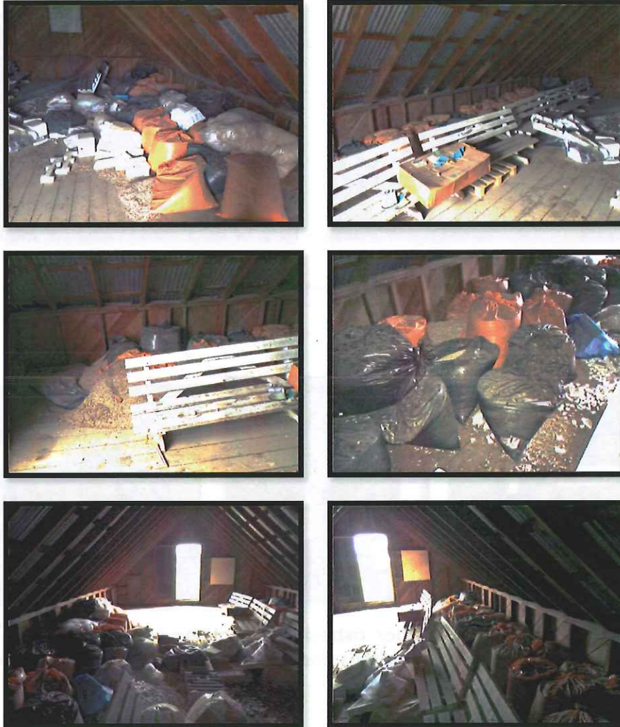
Photo Set 7 Building 50 – Attic space: asbestos-containing vermiculite insulation present in approximately 70 garbage bags as well as scattered throughout the attic – on the floor and on stored items
