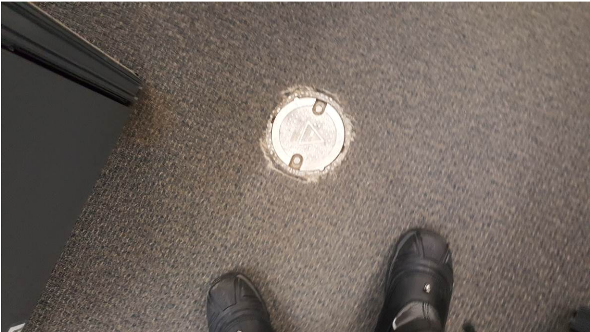
Photo 12 - Room - 1-120 - Floor Power
