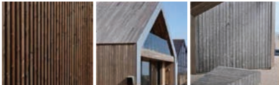
Distressed Wood Siding
