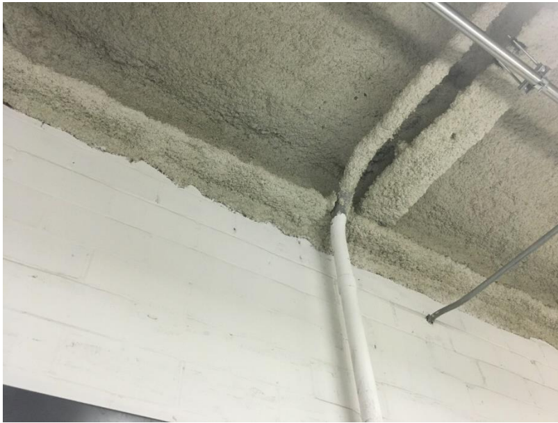
Photo 1: Non-friable asbestos-containing mortar associated with terracotta block throughout the project area. The sprayed fireproofing was confirmed to be non-ACM.
