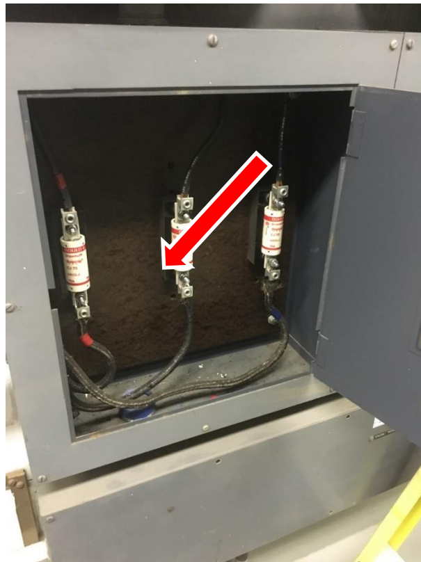
Photo 2: Assumed asbestos-containing Transite panels, located behind wall-mounted fuse boxes in the project area.
