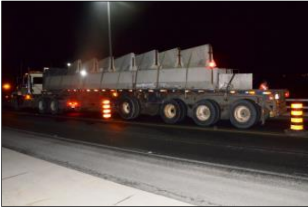
Fig 8: Truck used for load test on SB lane of bridge - Truck load=640 kN; Axle sp =4.3, 1.5, 6.5, 2.5, 1.5, 1.5 m
