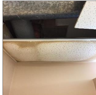
Photo # 8 - Mouldy ceiling tile finish within the office space.
