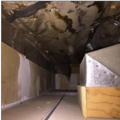
Photo # 7- Mouldy drywall, ceiling tile, and fibreglass batting within the kitchen.
