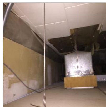
Photo # 2 - Non-asbestos wood cellulose mechanically fastened ceiling tiles present above lay-in tiles.
