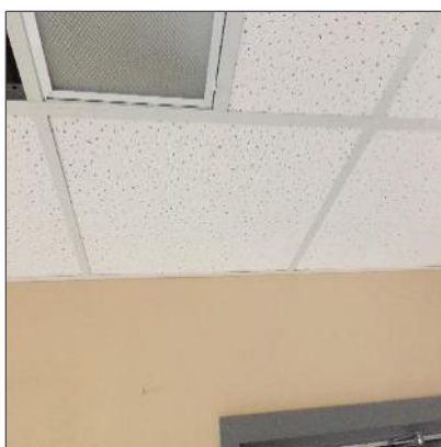
Photo # 1 - Non-asbestos acoustic ceiling tiles date stamped 1997 year of production.
