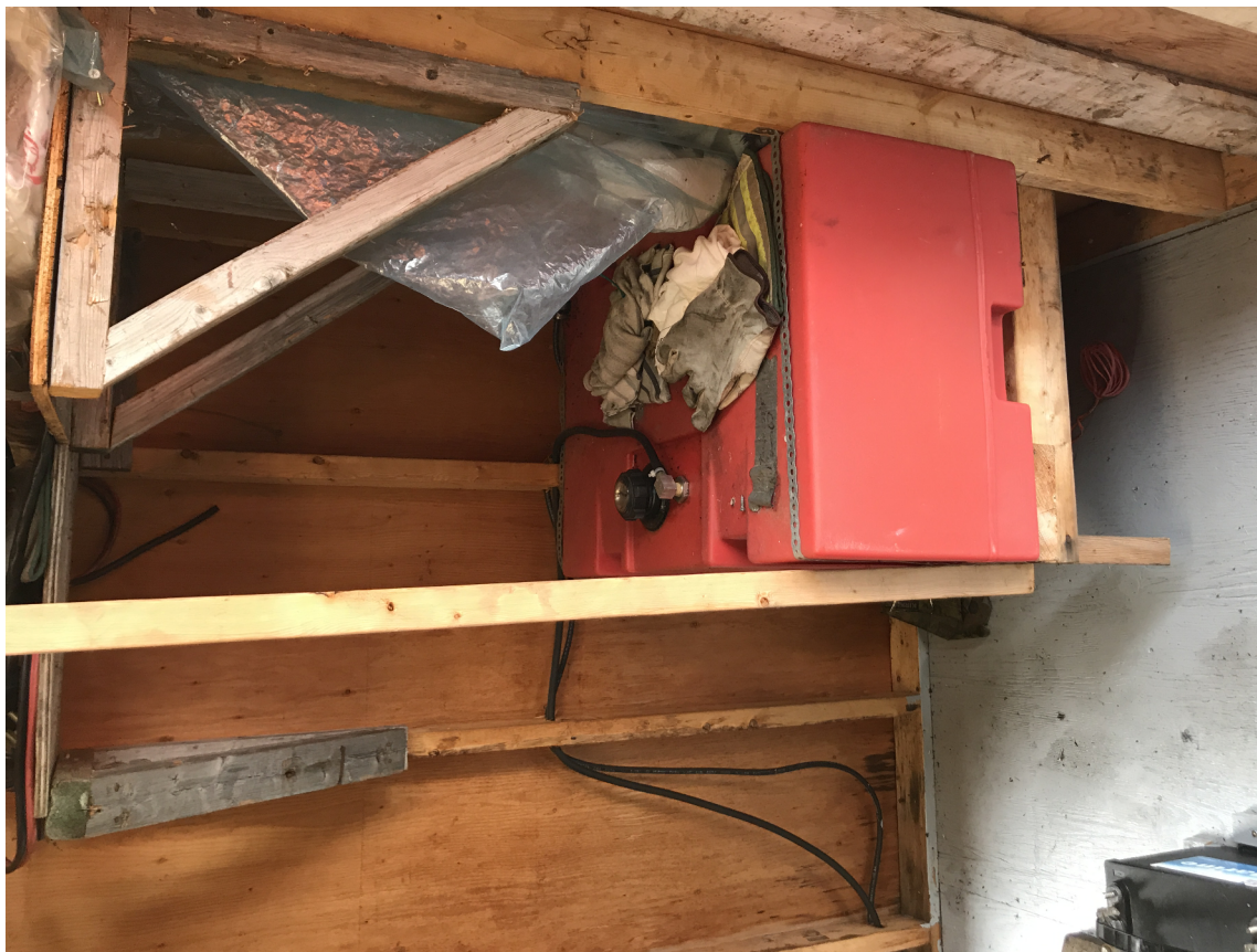
Generator Day Tank
