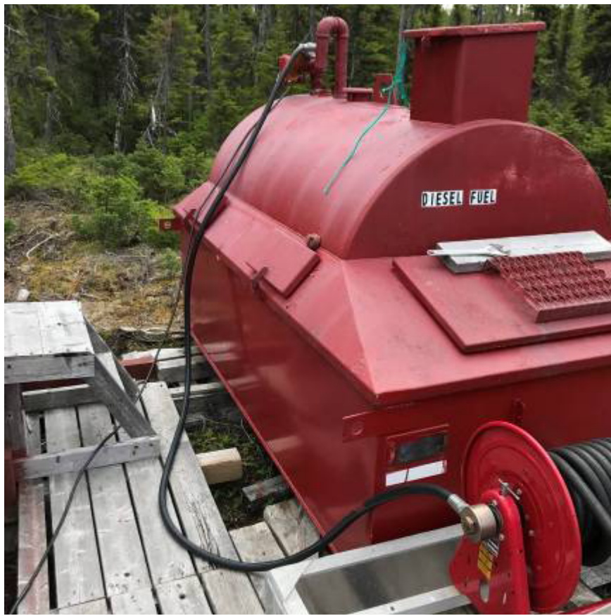
Fuel Tank Hose Reel and Pump Setup
