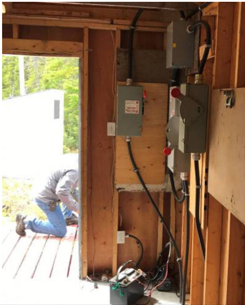
Generator House Electrical
