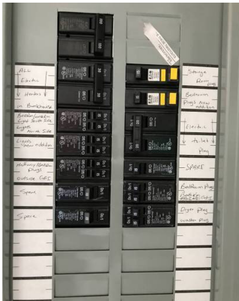
Bunk House Electrical Panel
