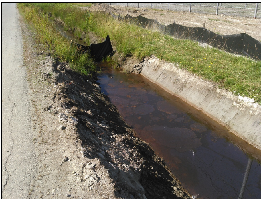
Photograph 13: Looking northeast at the headwall located in the ditch at 0+690 to be relocated and re-tied into the existing culvert during the proposed road works (July 11, 2017).
