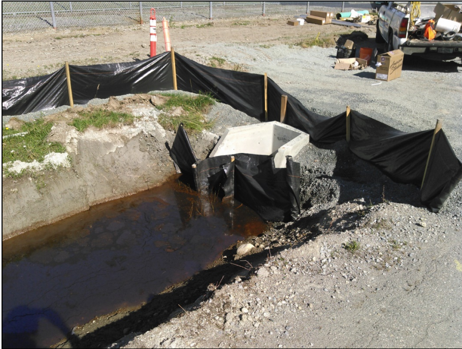
Photograph 11: Looking northeast at the headwall located at 0+690 in the ditch to be relocated and re-tied into the existing culvert during the proposed road works (July 11, 2017).
