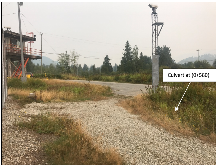
Photograph 6: Looking northeast of the culvert located at 0+580 in the ditch to be replaced during the proposed road works (September 7, 2017).
