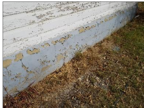
Photo 9. Grey, lead-containing exterior flaking foundation paint.
