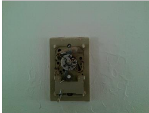
Photo 10. Thermostat in the hallway (Loc. 5) which contains mercury.
