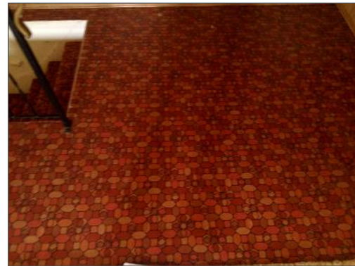
Photo 5. Asbestos-containing red vinyl sheet flooring on the 2 nd floor (Loc. 9).
