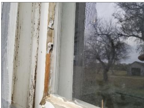
Photo 6. Asbestos-containing white caulking around exterior window frames.
