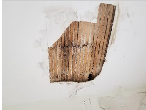
Photo 2. Non-asbestos containing plaster that has fallen away from the wood lath.
