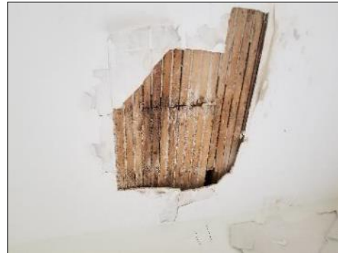
Photo 12. Ceiling mould and water damage on wood and plaster in the east bedroom (Loc. 6).
