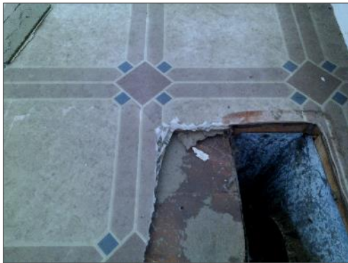
Photo 4. Asbestos-containing multi layered vinyl sheet flooring in the Kitchen (Loc. 3).
