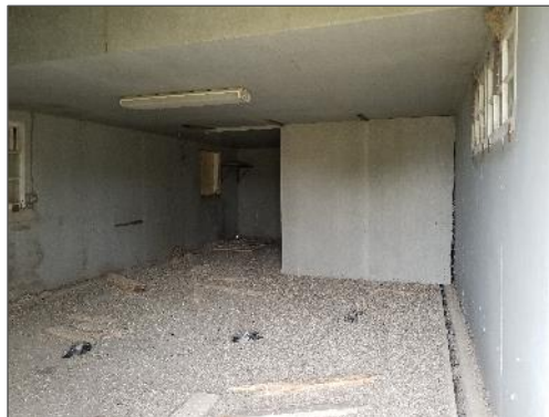
Photo 3. Transite board used for the walls and ceilings of the pigeon shack.
