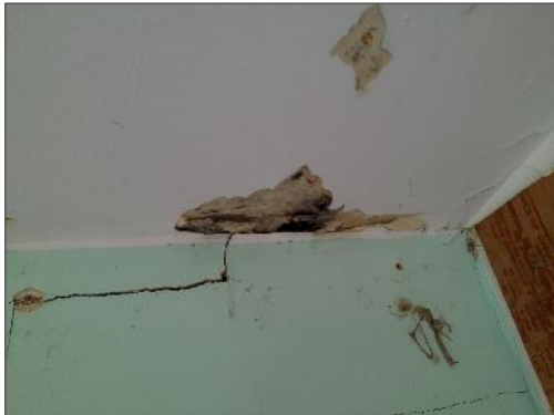
Photo 11. Ceiling mould in the front entrance (Loc. 2).
