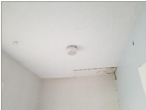
Photo 11. Ceiling mould in the west bedroom (Loc. 8).
