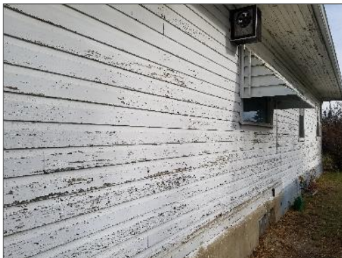
Photo 8. White, lead-containing exterior flaking white wall paint.
