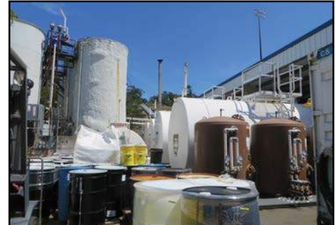
ADEQUATE containment of odorous waste.
