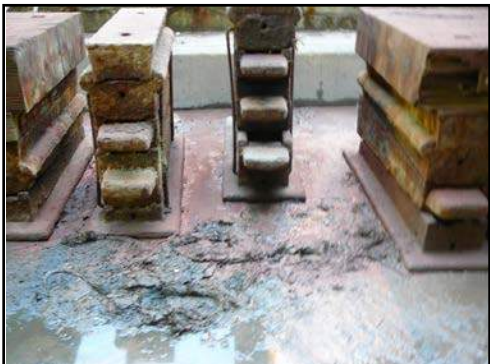
Sediment from the harbour often settles on dock bottom after dewatering. If this becomes contaminated with paint, etc., it must be disposed of.
