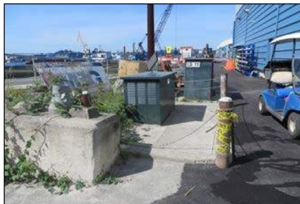
AUTHORIZED Sanitary Sewer Discharge point, Lift Station #11.
