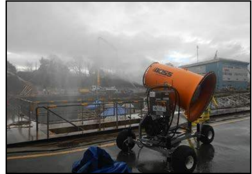
Dust suppression unit in operation.
