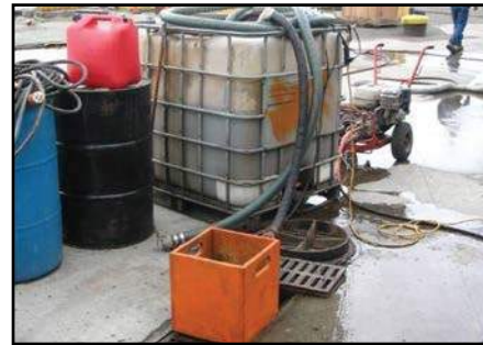
The trench drain is blocked and a sump pump is installed to collect wash water into a tote.
