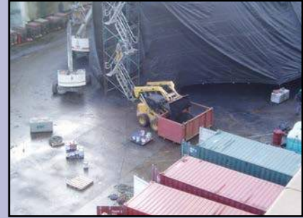
Remove waste grit from work areas as soon as possible to prevent migration of contaminants throughout the drydock floor.
