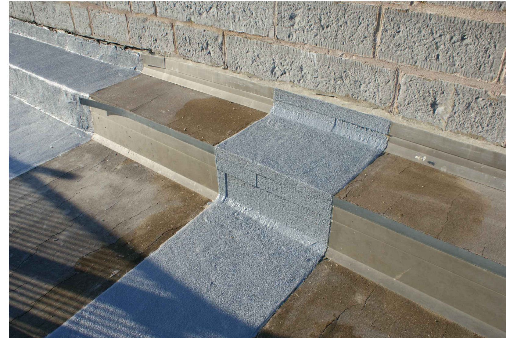
MOCK UP OVER EXISTING MASTIC ASPHALT AND STEEL FLASHING AT STONE FIRING STEPS N.T.S.
