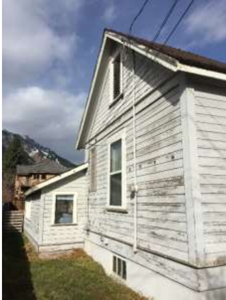
Exterior paint on the structure that was analyzed to have excessive lead content.
