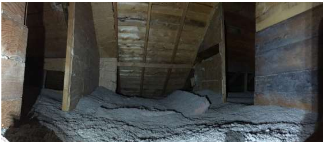
Vermiculite insulation is located beneath the batt and cellulose insulation. Attic space is compartmentalized into four areas, three of the areas are shown in this photo
