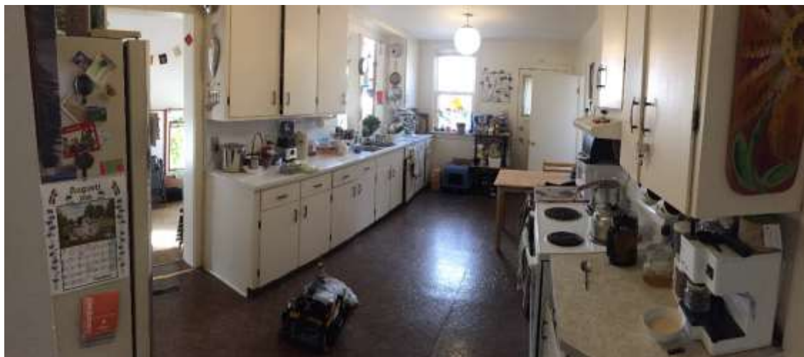
Identified asbestos containing brown linoleum flooring within the kitchen
