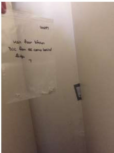
Drywall sample location with the positive asbestos identification.
