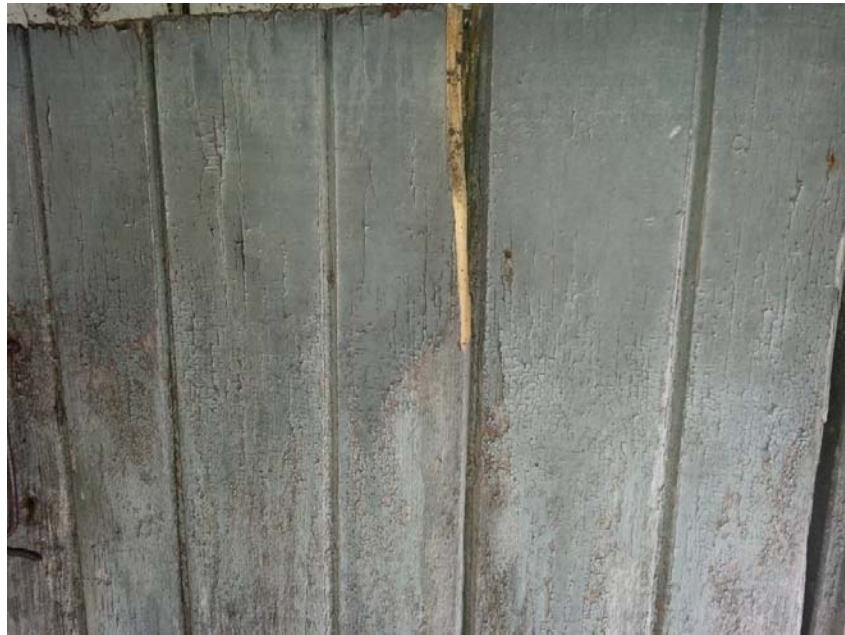
Photo 7: View of lead based grey door paint in building 97516. Sample P-01.
