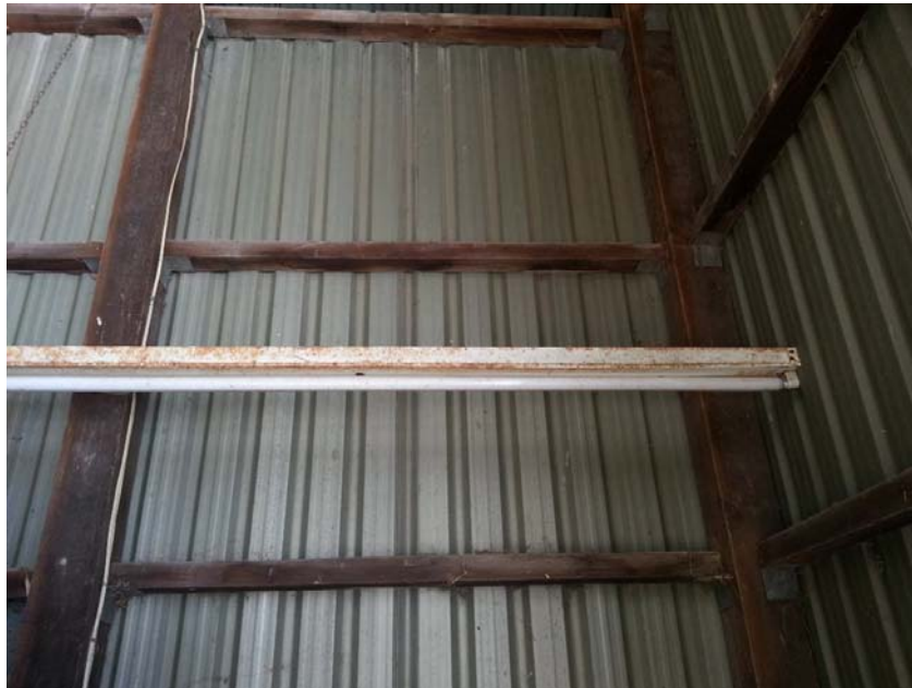
Photo 10: View of mercury containing fluorescent light tube and potential PCB containing ballast in building 3347.
