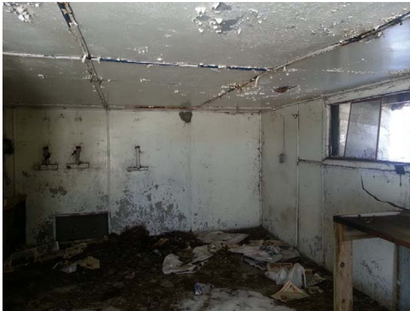
Photo 6: View of asbestos containing transite cement board in building asset 97514. Sample set T-01A-C. As well as lead containing white wall paint. Sample P-03.
