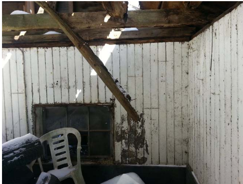
Photo 8: View of lead based white wall paint in building 97516. Sample P-02.
