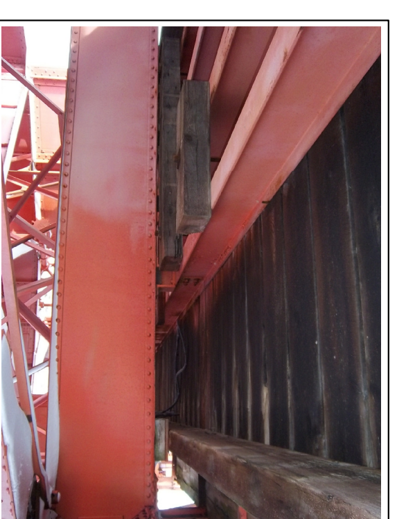
8 REPLACE EXISTING EQUIPMENT ANCHORS & SANDBLAST AND PAINT ALL PAINTED SURFACES - EQUIPMENT ACCESSIBLE AFTER DECK REPLACEMENT
