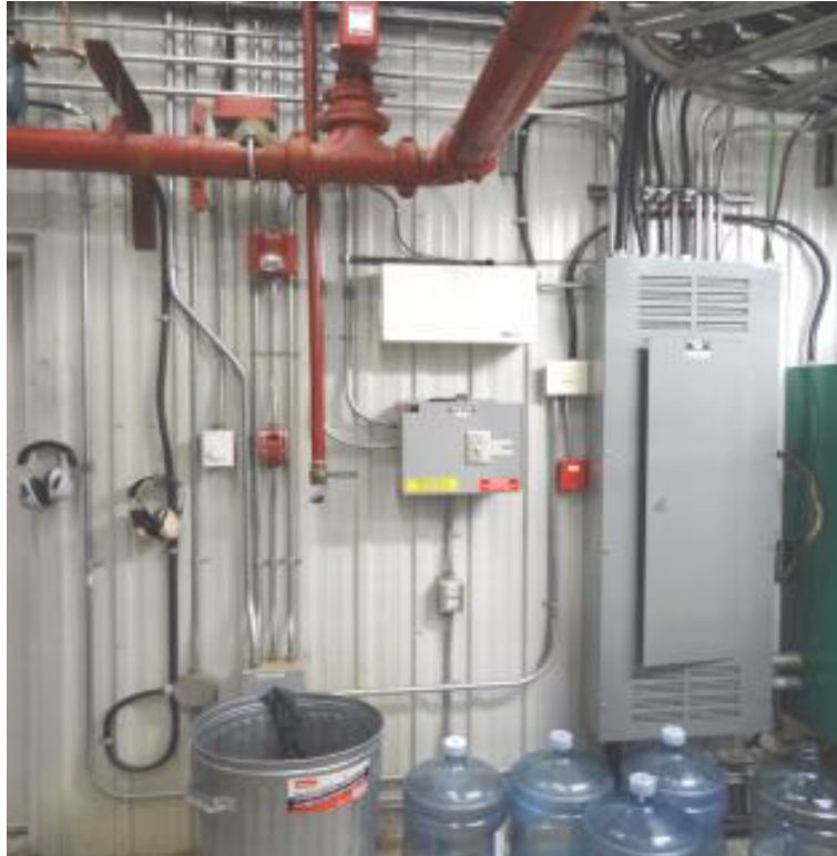
Existing Panelboard A
