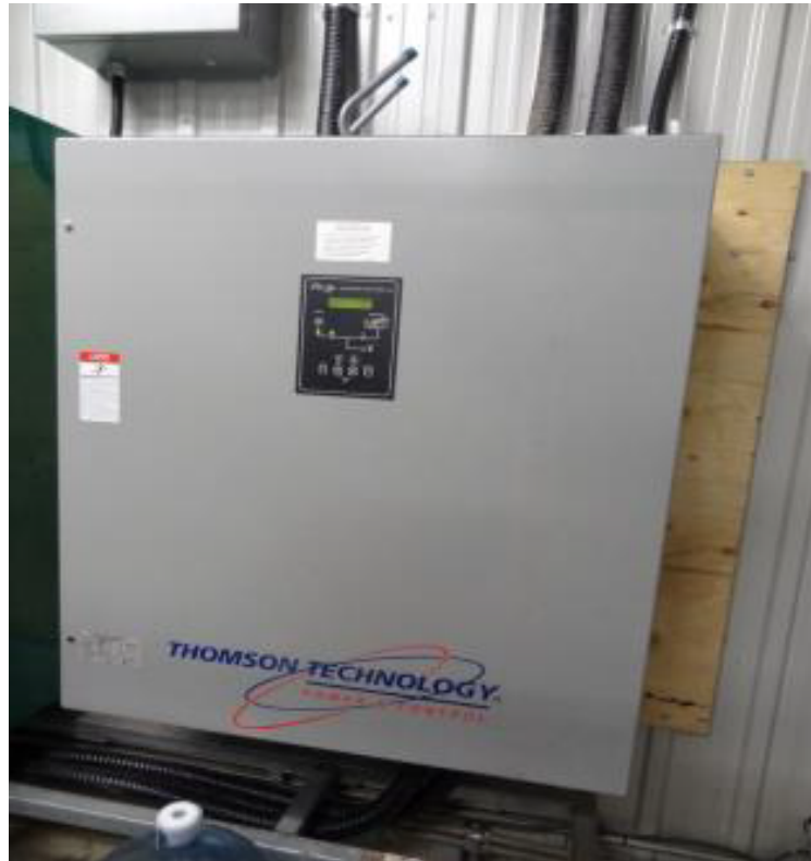
Existing Thomson Technology Transfer Switch
