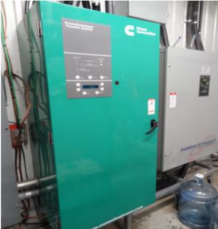
Existing Cummins Automatic Transfer Switch
