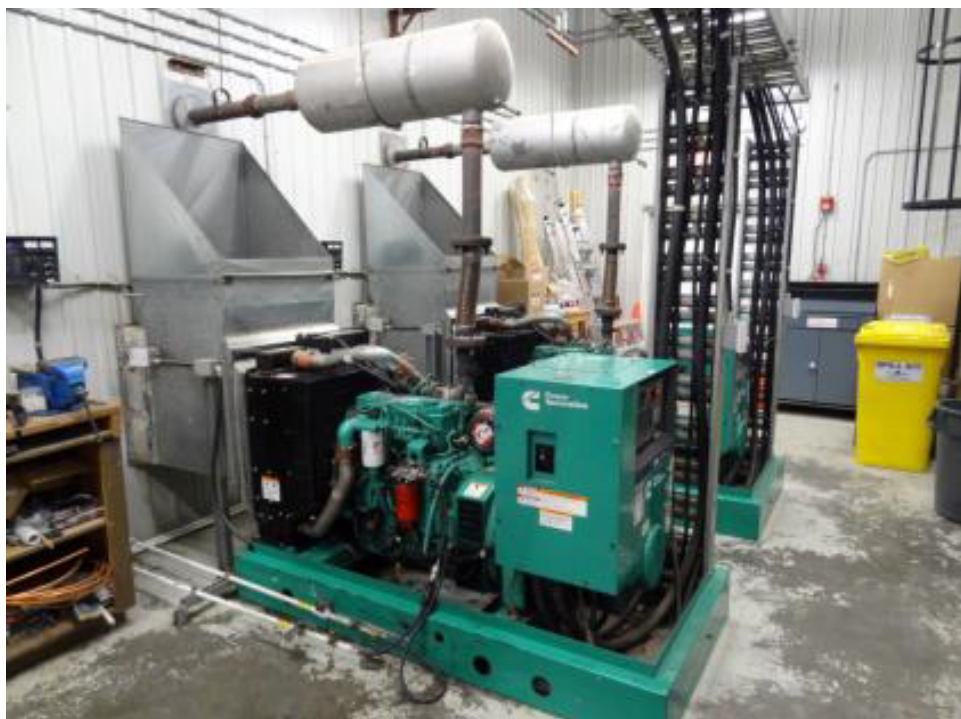
Existing 72kW Generators
