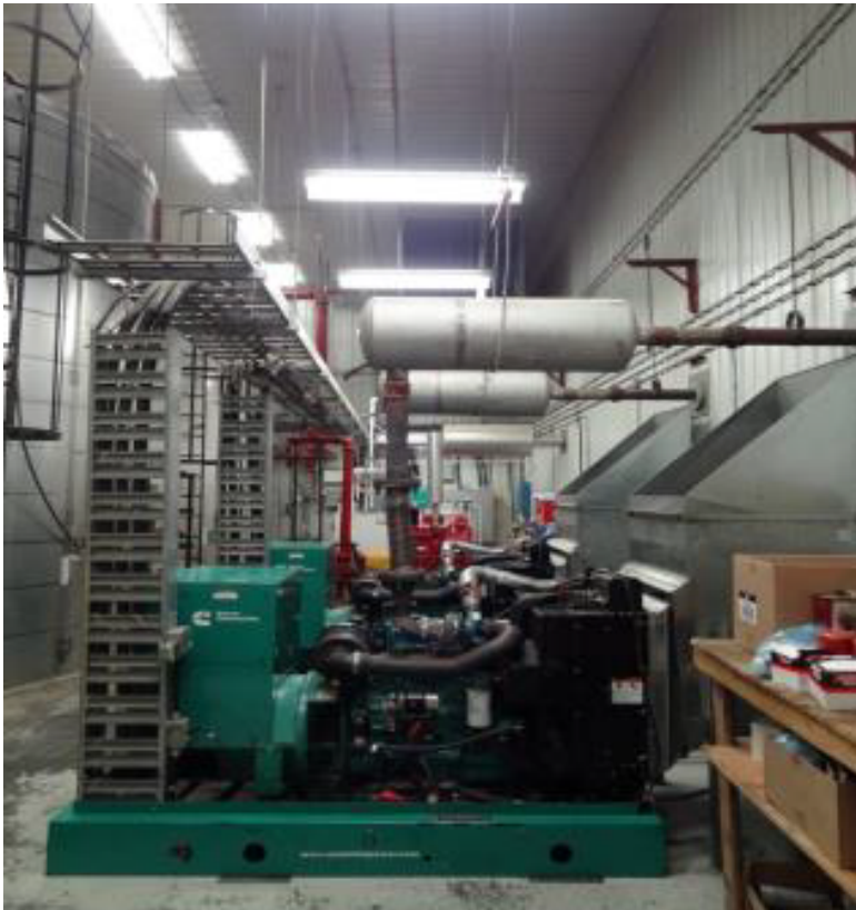
Existing 72kW Generators
