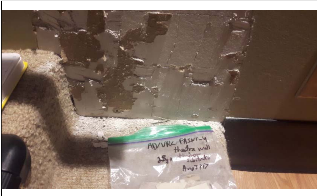
Photo 16: AD/VRC-Paint 4, Interior Wall of Theatre in Admin/VRC Building
