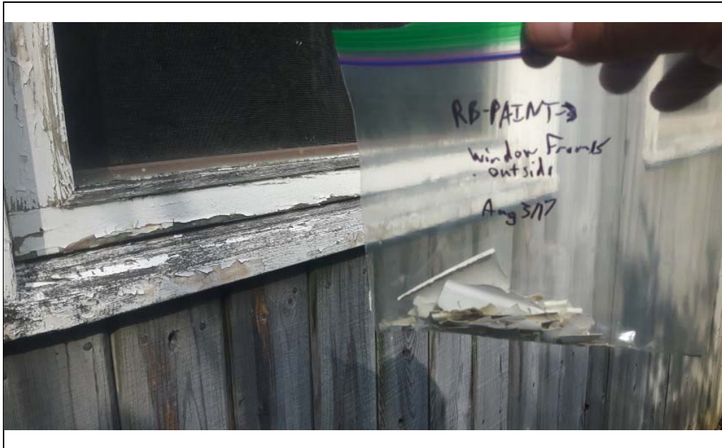
Photo 12: RB-Paint-3, Exterior window trim
