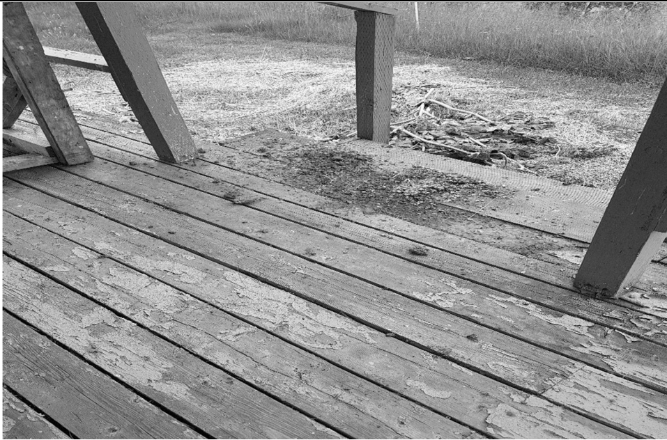
Photo 9 Date: July 13, 2017 Location: BFF Campsite - Cabins Description: Typical view of the built-up avian guano on the wooden steps of the cabin.
