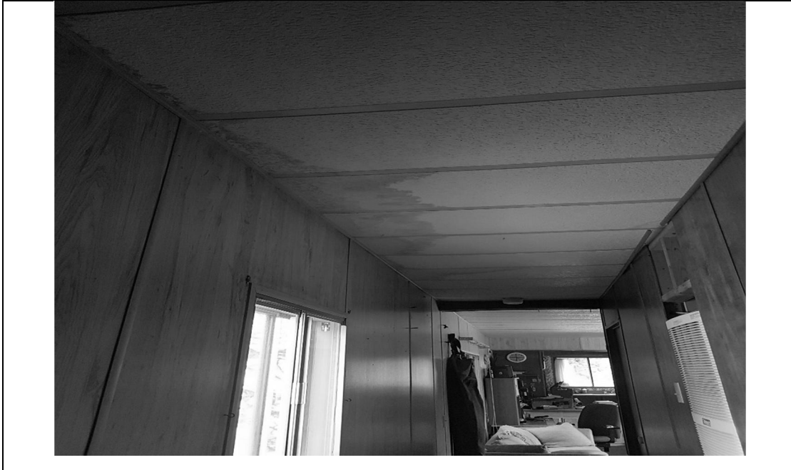
Photo 5 Date: July 13, 2017 Location: BFF Campsite - Trailer Description: View of the perimeter surface staining of the ceiling. Cause is water seepage through the roof.
