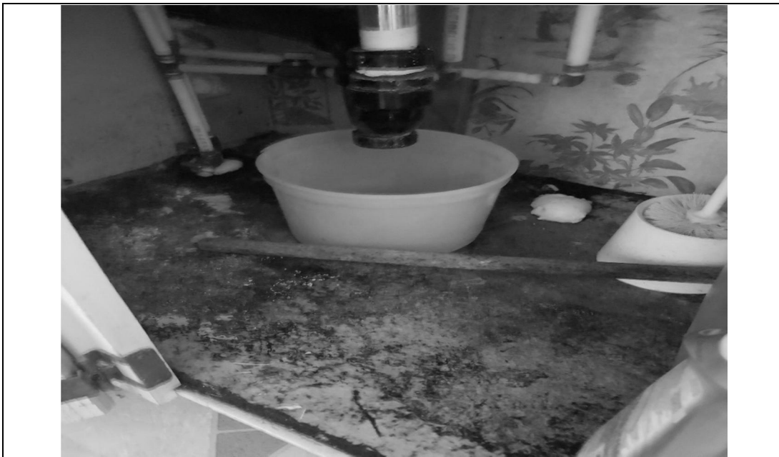
Photo 6 Date: July 13, 2017 Location: BFF Campsite - Trailer Description: View of the bathroom sink cabinet; suspect fungal growth on surface of cabinet.
