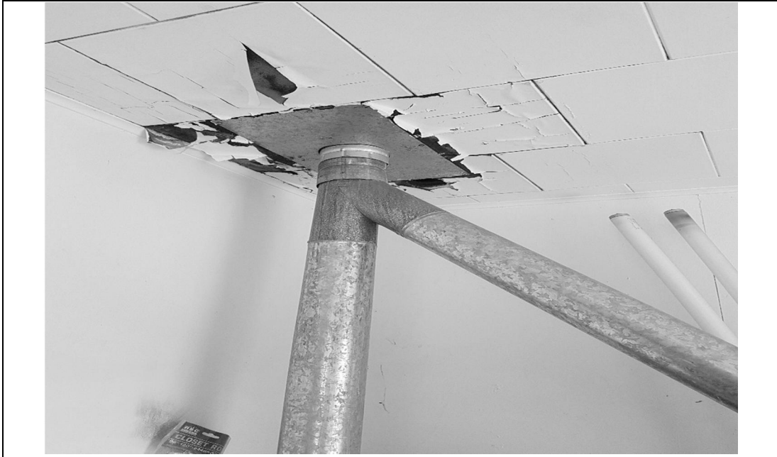
Photo 7 Date: July 13, 2017 Location: BFF Campsite - Kitchen Description: View of the suspect fungal growth on ceiling tiles in Laundry Room.
