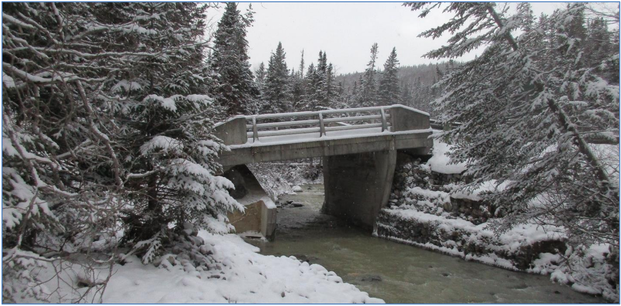
Figure 2. Damaged bridge crossing Barters Brook along the access road to Lomond Campground; this bridge was removed in February 2018.
