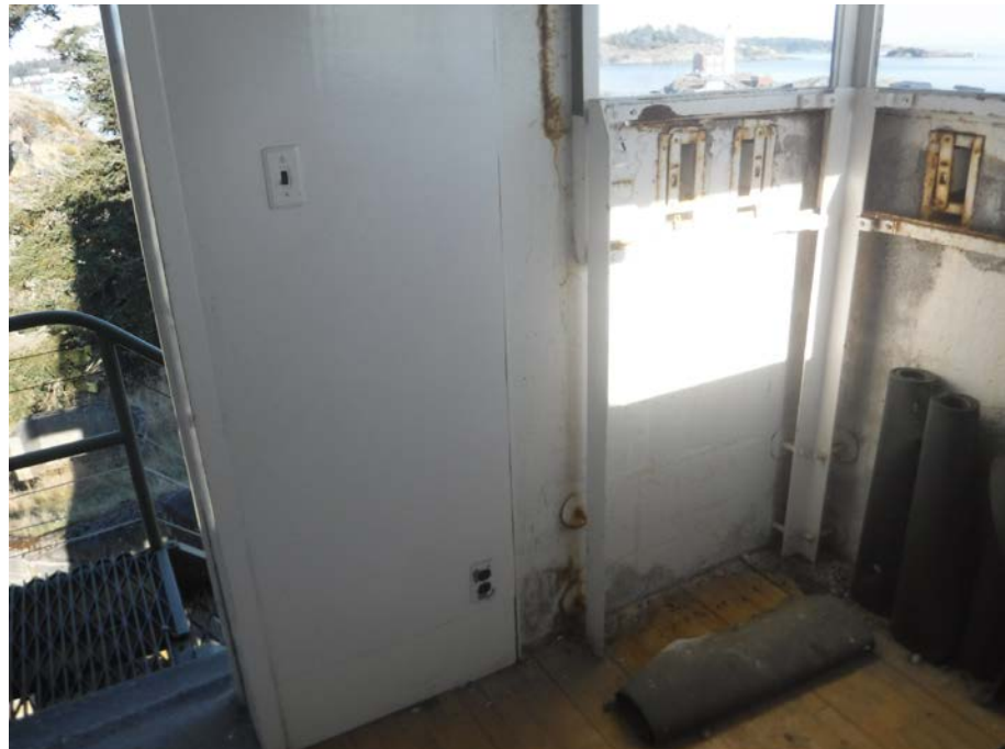
Photo 28: Interior surface of wall pier covered in wood panels and exposed concrete below window
