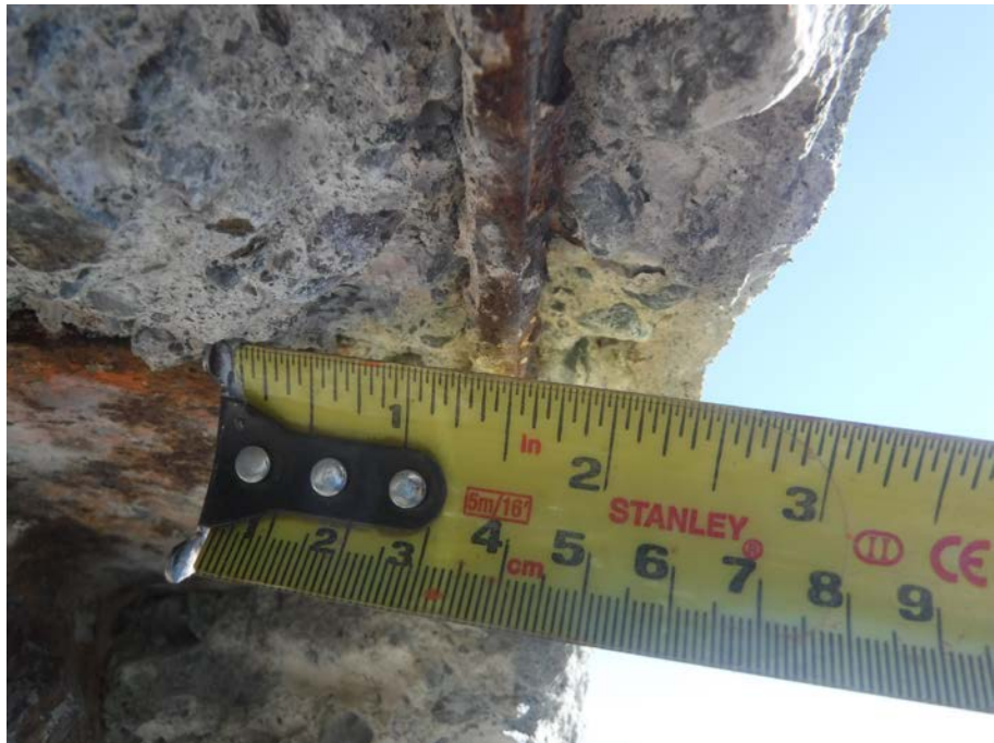
Photo 20: Horizontal reinforcement exposed in northwest leg
