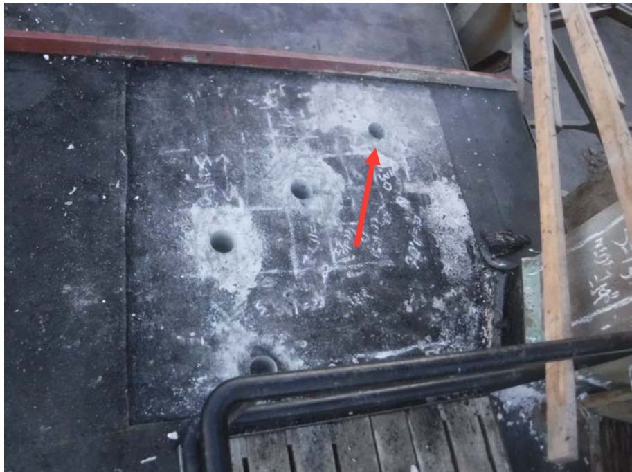
Photo 24: Location of cut rebar
