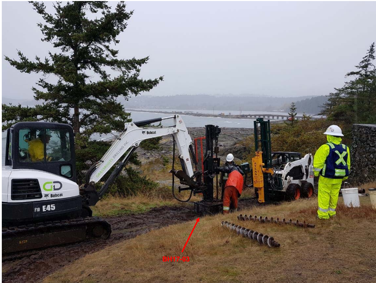
Photograph 6: Approximate location of the second borehole at the west Belmont Retaining Wall. Photograph also displays the limited access drilling equipment used in this area.
