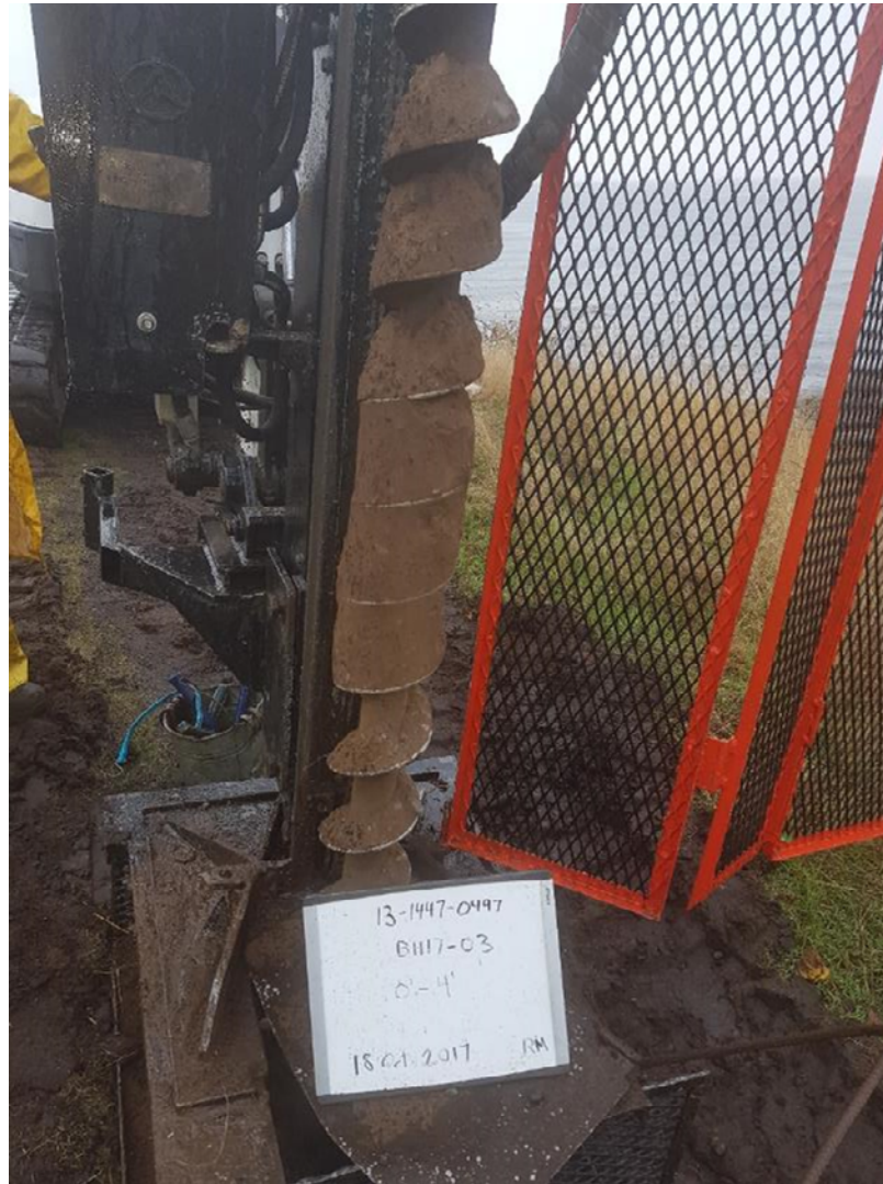
Photograph 7: Example of silty sand fill material from BH17-03 at the west Belmont Retaining Wall
