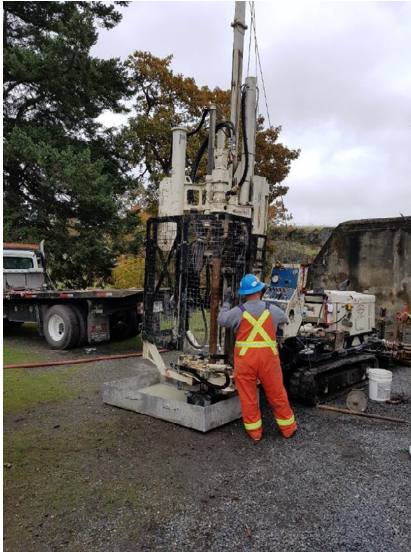
Photograph 2: Track-mounted drill rig used at the Belmont Director's Tower and the Lower Battery Underground Magazine
