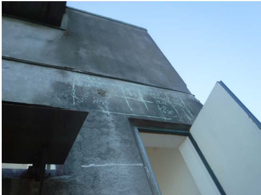
Photo 14: Door frame limits GPR access to floor beam underside
