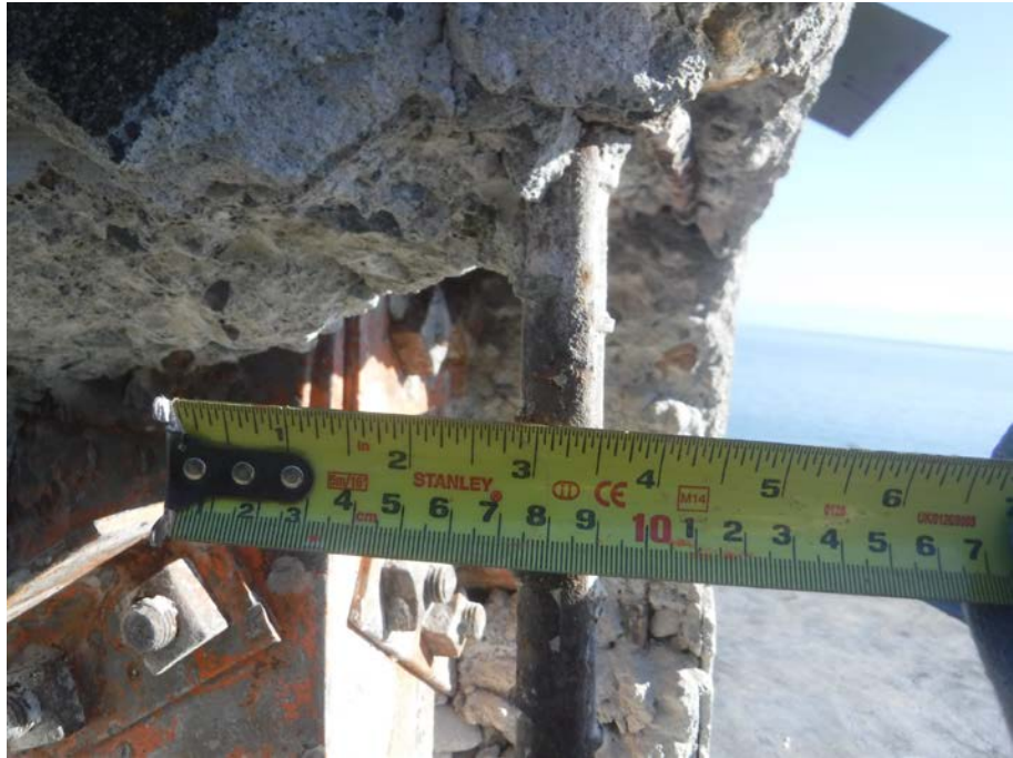
Photo 19: Vertical reinforcement exposed in northwest leg
