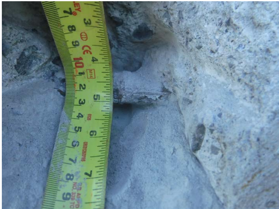
Photo 16: Horizontal reinforcement exposed
