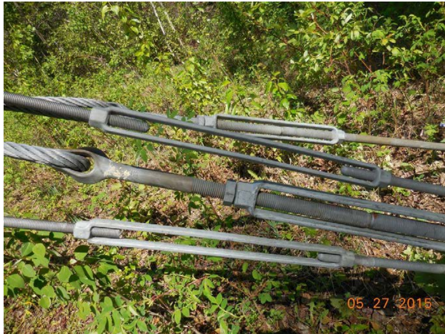
Photograph 3: Typical cable turnbuckle arrangement.
