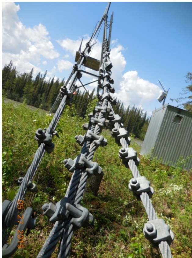
Photograph 4: Typical clip-type cable terminations.
