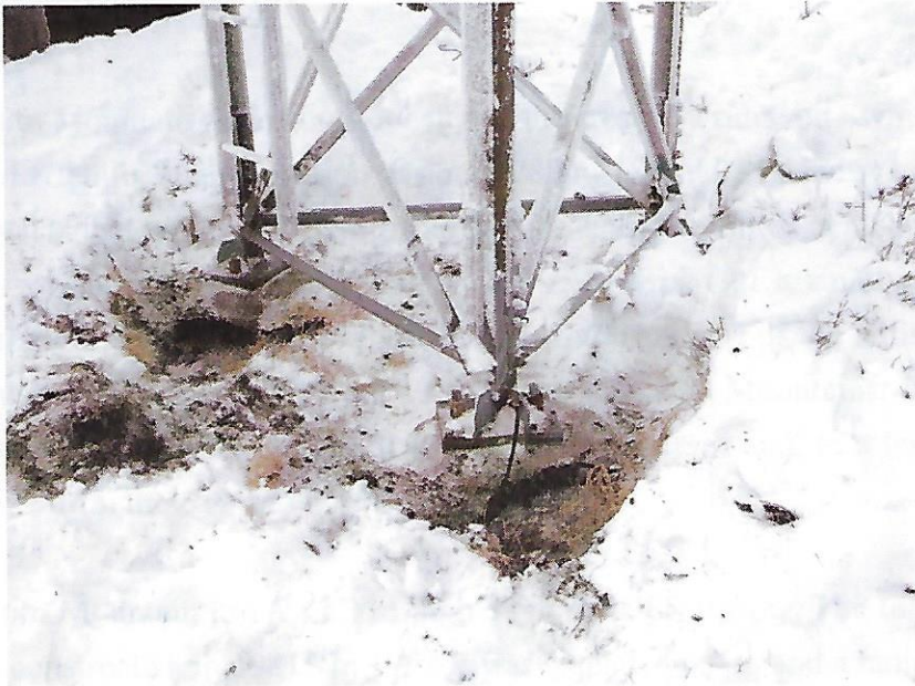
Photo K1711-Mount Gil-01: View southwest to tower. Note regular surface of snow and low grout pads that footings are set on. Slope across site here is very gently dipping to northwest and is relatively flat. Topsoil in excavations was 75 to 125 mm thickness.
