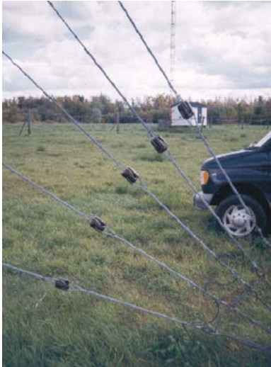
Figure 2-4 shows part of the base section of an old 220 feet (67 m) isolated tower sitting on top of the insulator. The spark gap arrester has to have its contact balls positioned horizontally to prevent water from shortening the gap. Figure 2-5 shows isolated guys.
