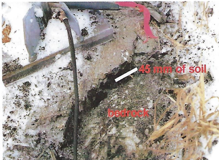
Photo K1711-Mount Gil-02: The foundations consist of steel plates set on grout pads with two Dywidag bolts penetrating rock 2.44 m. Bolts size are #8 Dywidag and length is 2.44 m according to the 1992 assessment. Note peaty soil between grout pad and bedrock. Soil thickness, if any, directly beneath the steel pad and grout is unknown.
