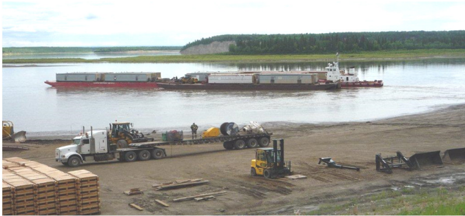
Cooper Barging Service Fort Simpson terminal near the junction of Mackenzie Highway 1 and Liard Highway 7.
