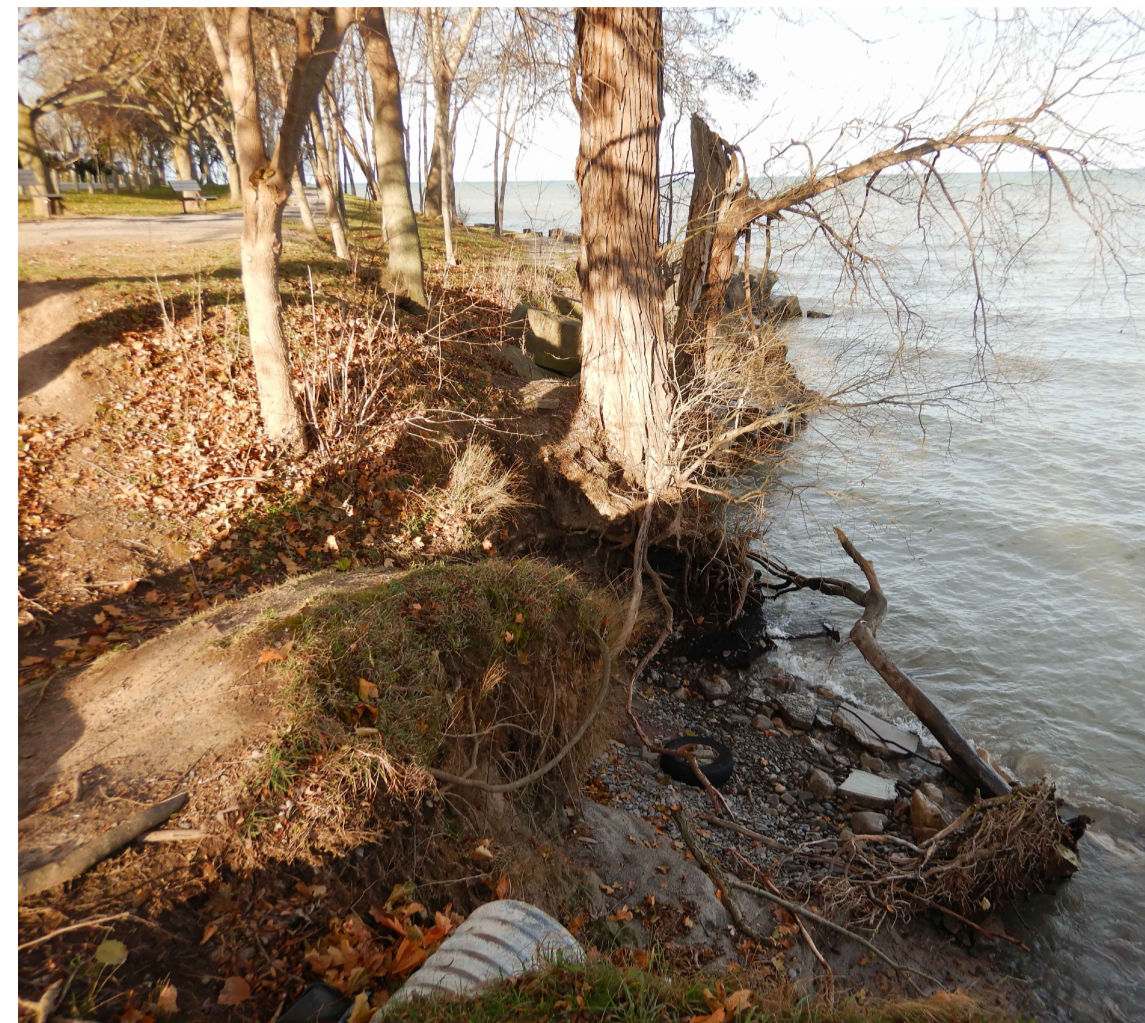
PHOTO 7 - WEST OF WORK SITE NEAR CHAINAGE 0+020 INCLUDING PLUGGED CORRUGATED PIPE
