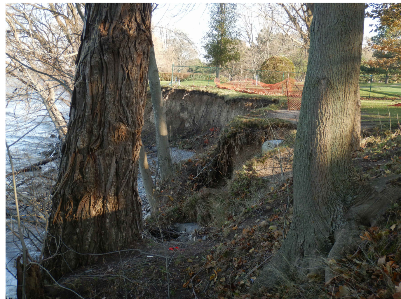
PHOTO 8 - WEST OF WORK SITE NEAR CHAINAGE 0+000 INCLUDING PLUGGED CORRUGATED PIPE
