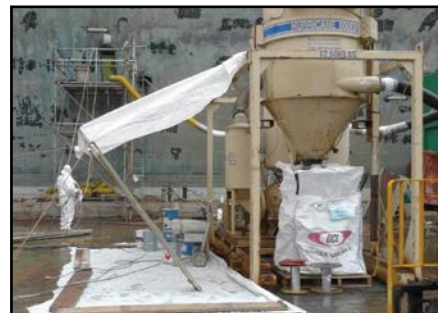
All hazardous materials must be stored in appropriate containment and away from tunnel drain system.
