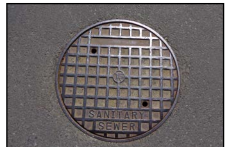
UNAUTHORIZED Sanitary Sewer Discharge point (i.e. sewer manhole).
