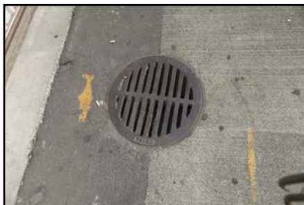
UNAUTHORIZED Sanitary Sewer Discharge point (i.e. storm drain).
