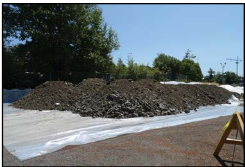
INADEQUATE stockpile of contaminated soil. Soil should be covered to prevent exposure to elements, runoff and people.
