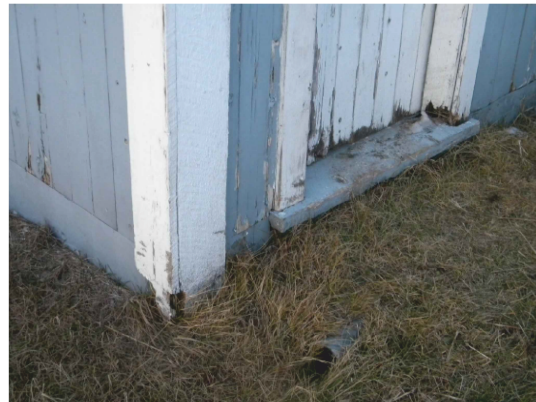
PHOTO 2 - EXISTING CORNER MOLDING
