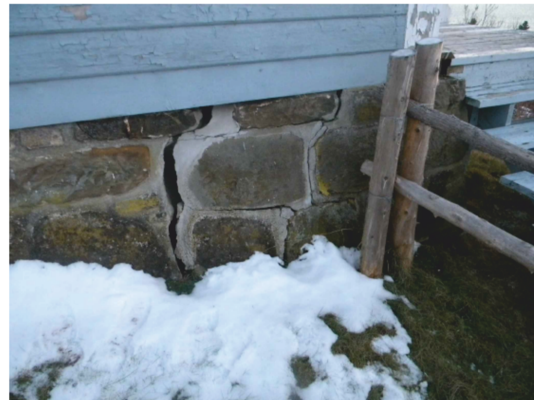
PHOTO 1 - EXISTING CRACKED FOUNDATION
