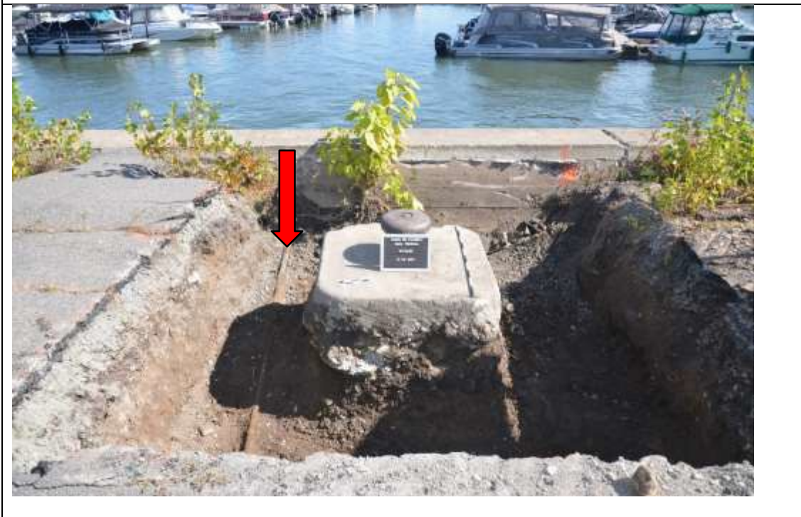
Figure 8 – Size of excavation, bollard, massive concrete base and tie attached to wall (510G13C102) located in the southeastern part of the Federal Wharf (Photo Matthieu Paradis, Parks Canada).
