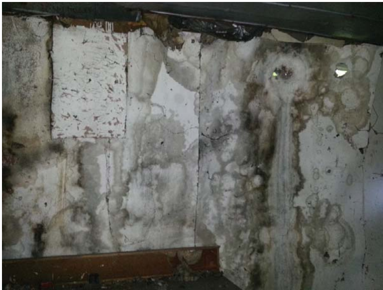
Photo 3: View of water damage and suspected mould growth in Building 1.
