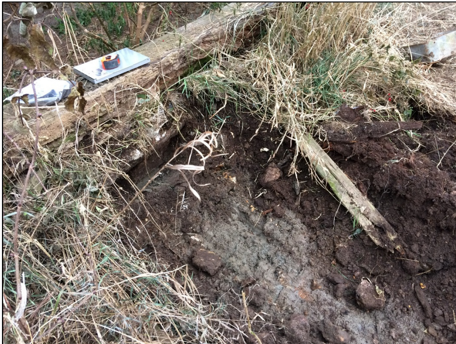
Photo 2: Exterior of Building 'A', showing wooden grade beam placed on top of dry stacked rock wedge foundation. The native glacial till is visible as the lighter brown material.
