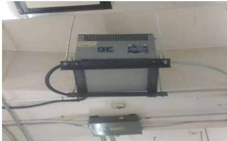
Figure 3-3 Existing Ceiling-Mounted Transformer used for the Primero PL-1840 Lathe
