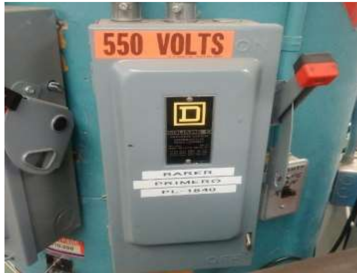
Figure 3-2 Existing Disconnect Box used for the Primero PL-1840 Lathe
