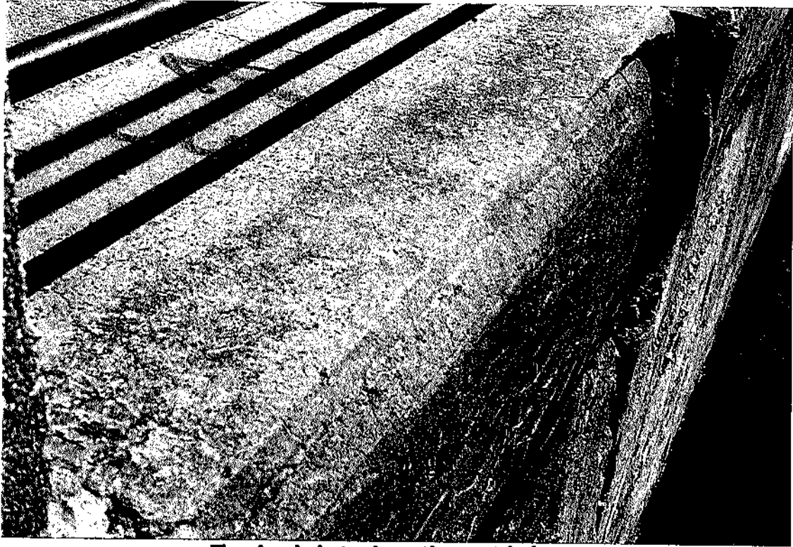
Typical deterioration at joint, close to B.H. 103
