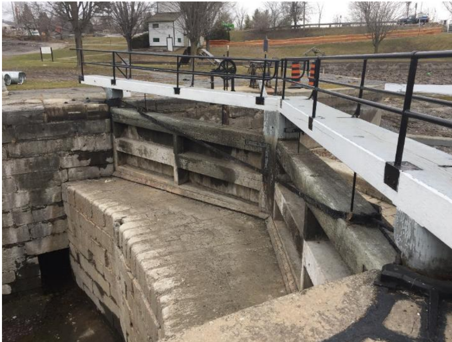
Photo 1: View of lock 47 upper gate, looking northwest. Black, grey, and white paints, located on the wood gates, as well as black paints located on the metal structures, including the railings, were found to be lead containing (DST Samples KM-LP-01, KM-LP-02, and KM-LP-03).
