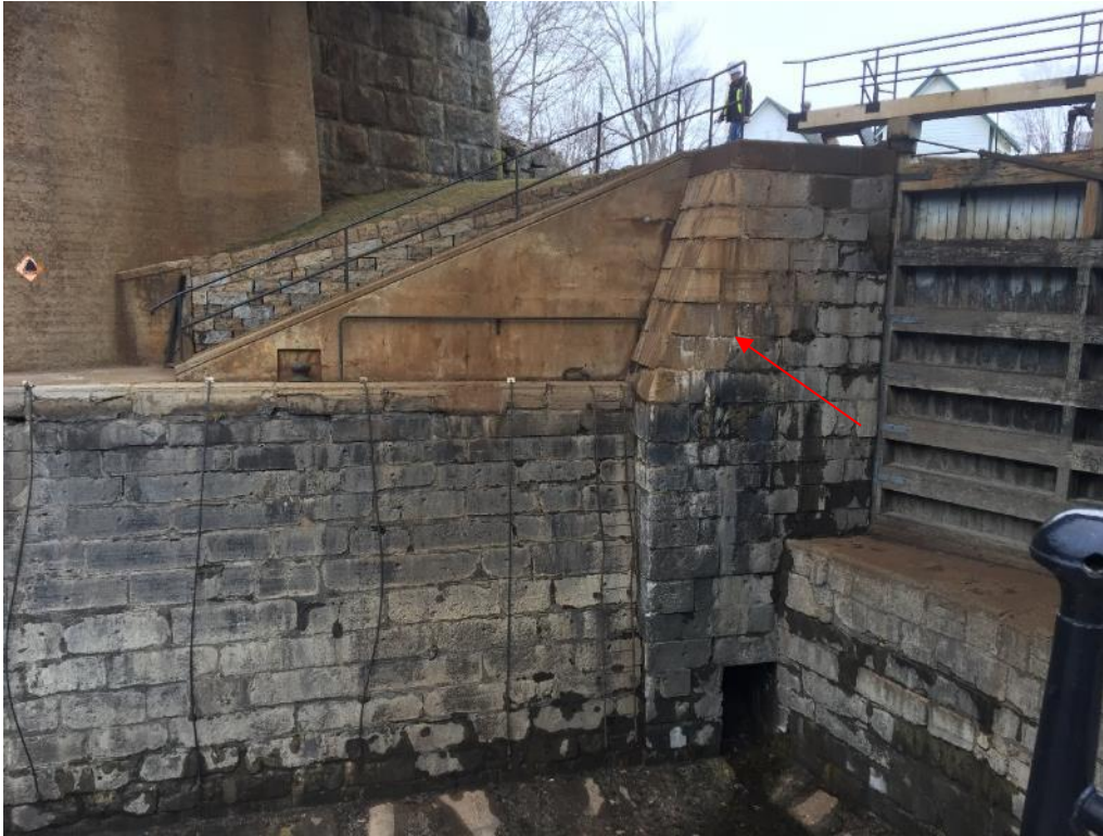
Photo 5: View of rust staining and debris from overhead rail bridge, located on the upper gate of lock 48 and lower gate of lock 47.
