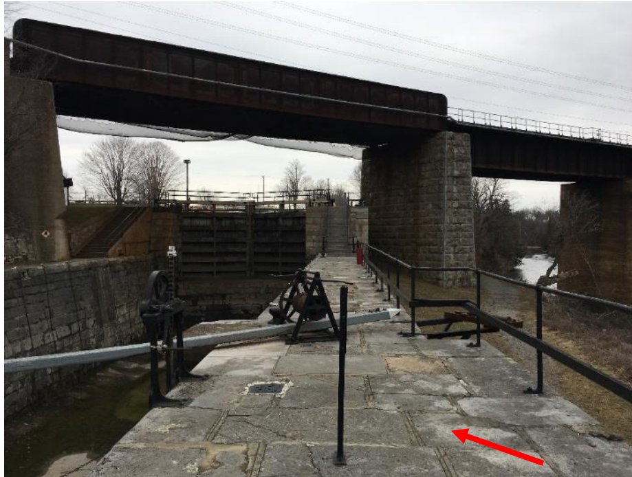
Photo 3: View of lock 48 upper gates, looking north. Concrete mortar (older) (DST Samples KM-02A-E), non-detect for asbestos, located on the basin walls.
