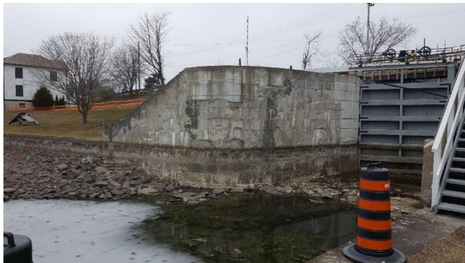
Photo 4: View of lock 46 lower gate, concrete blocks and mortar (newer) (DST Samples KM-03A-C, respectively), non-detect for asbestos, looking north
