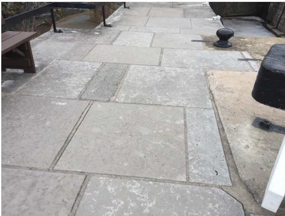
Photo 2: View of concrete blocks and mortar (DST Samples KM-04A-C and KM-01A-C, respectively), located on the eastern portion of lock 47, found to be non-detect for asbestos
