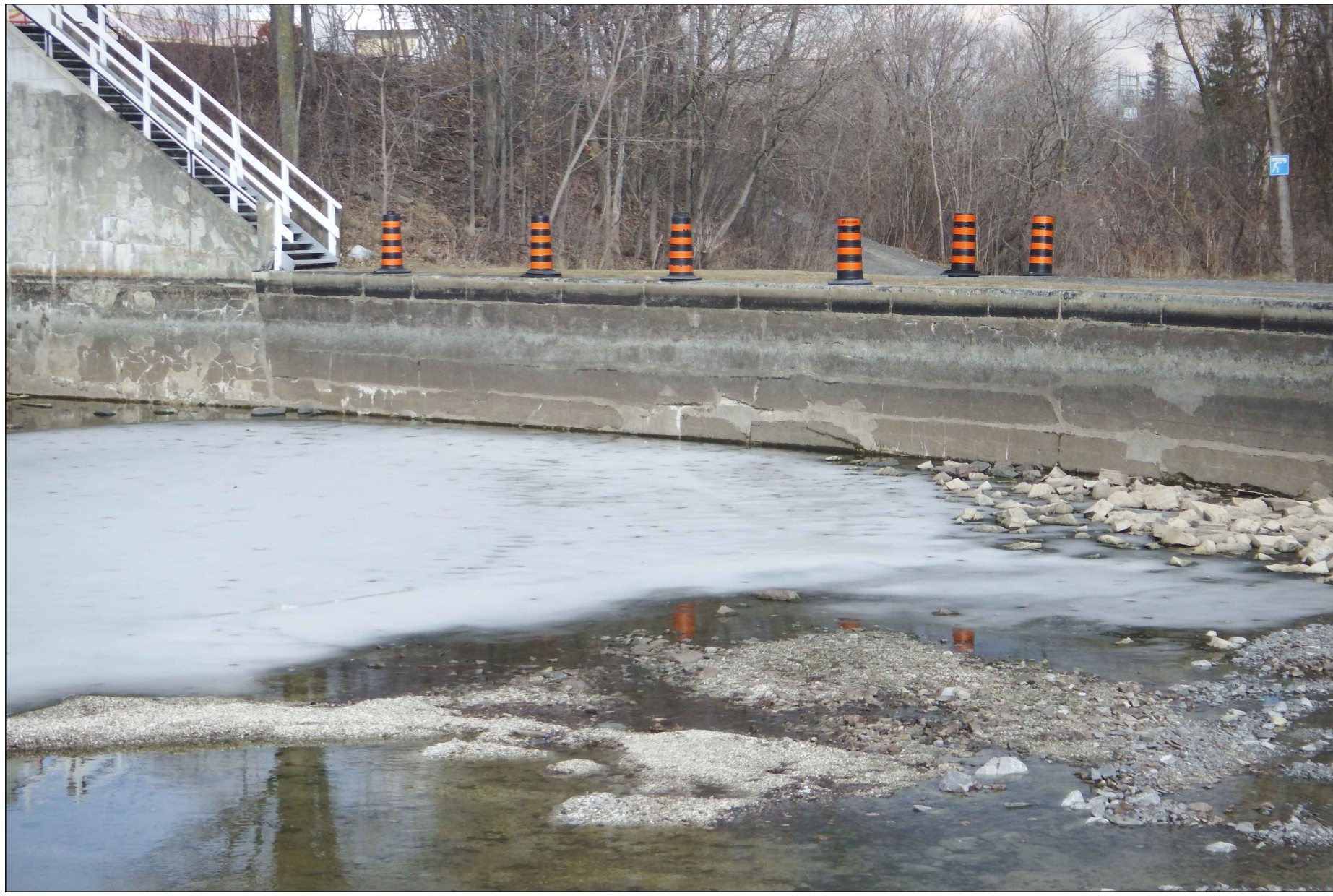
EAST BASIN WALL (NORTH END) - 2017
