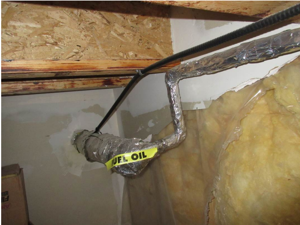
Photo 11 FUEL PIPE ENTRY INTO CRAWL SPACE
