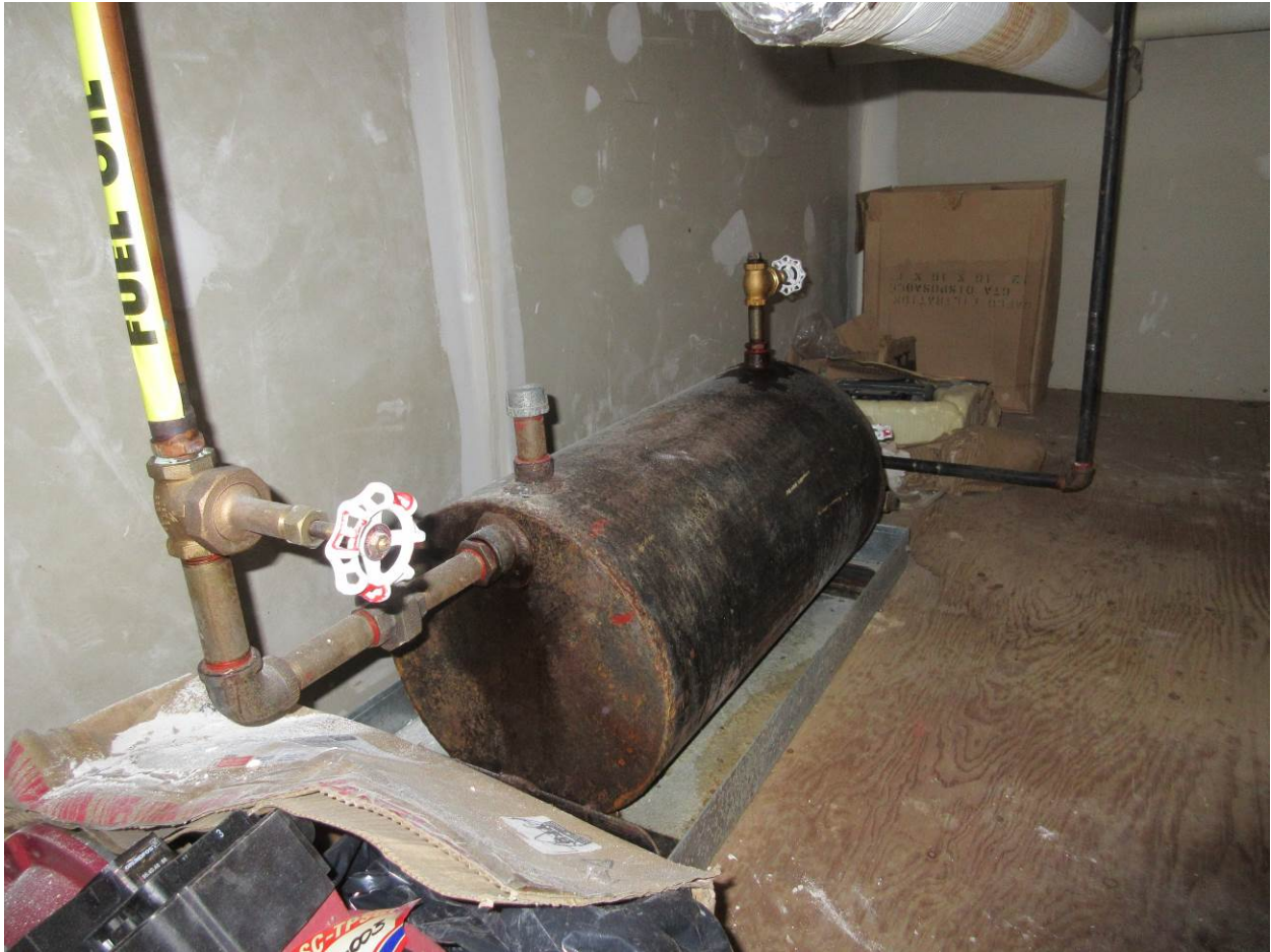
Photo 13 INTERIOR DAY TANK – BOILERS
