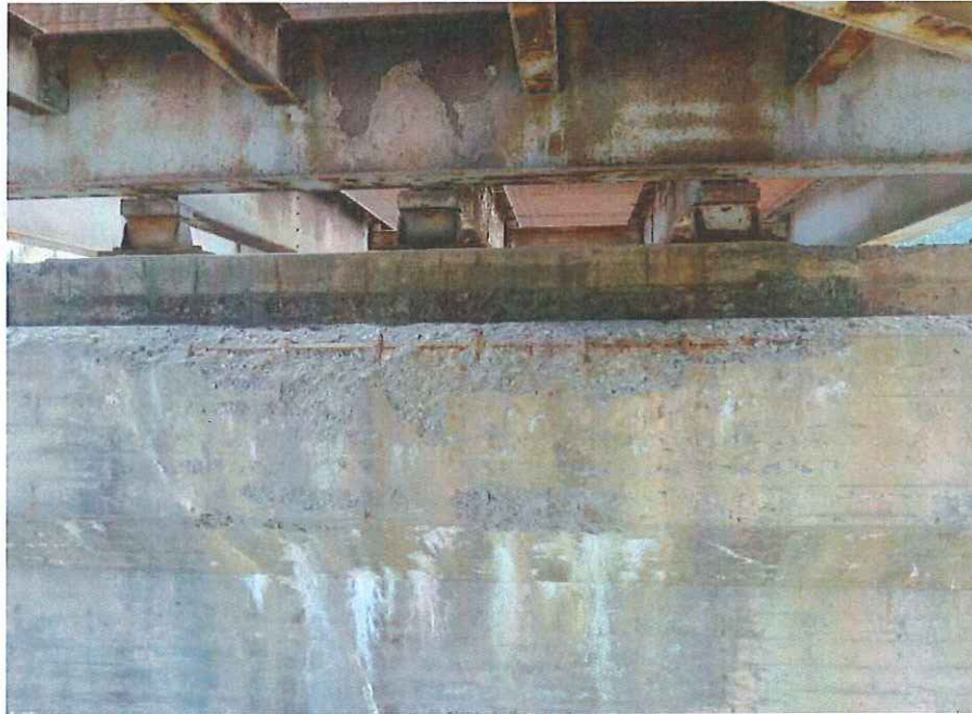
P23 - Spalls and leaching cracks on N face of S Pier
