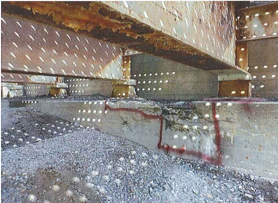
P18 - Spalls on face of N Abutment beneath girder bearing
