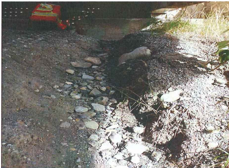
P40 - Erosion of material deposited from roadway onto N embankment beneath Span 3
