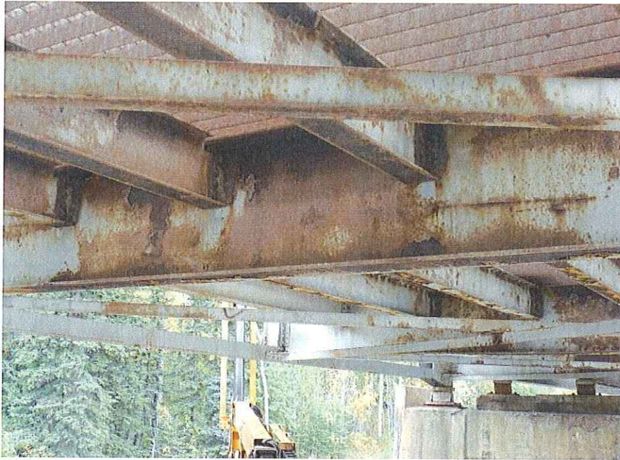
P57 - Typical condition of steel coating on steel floor beams and stringers on Span 2
