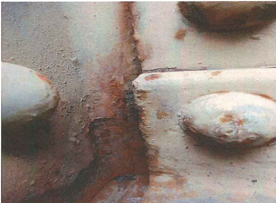
P32 - Cracking in steel at E side of end post at N end of W truss
