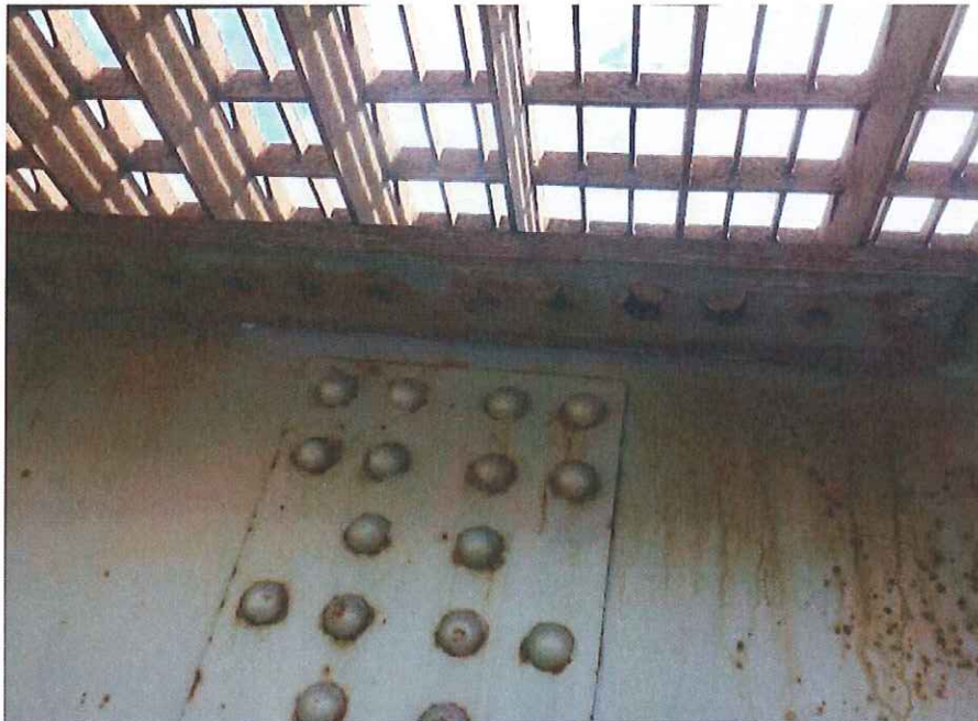
P39 - Missing rivets in top flange splice on W side of Girder G1 in Span 3
