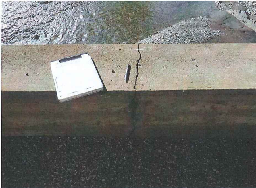
P27 - Wide vertical crack in middle of wall at base of N Pier
