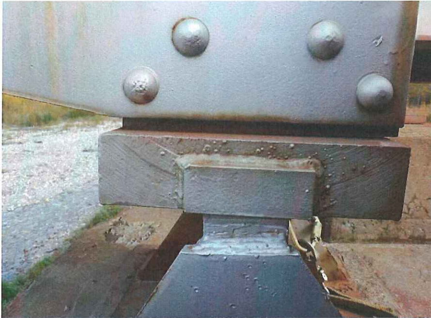
P35 - Gap between W flange on end post and bearing top plate at S end of W truss
