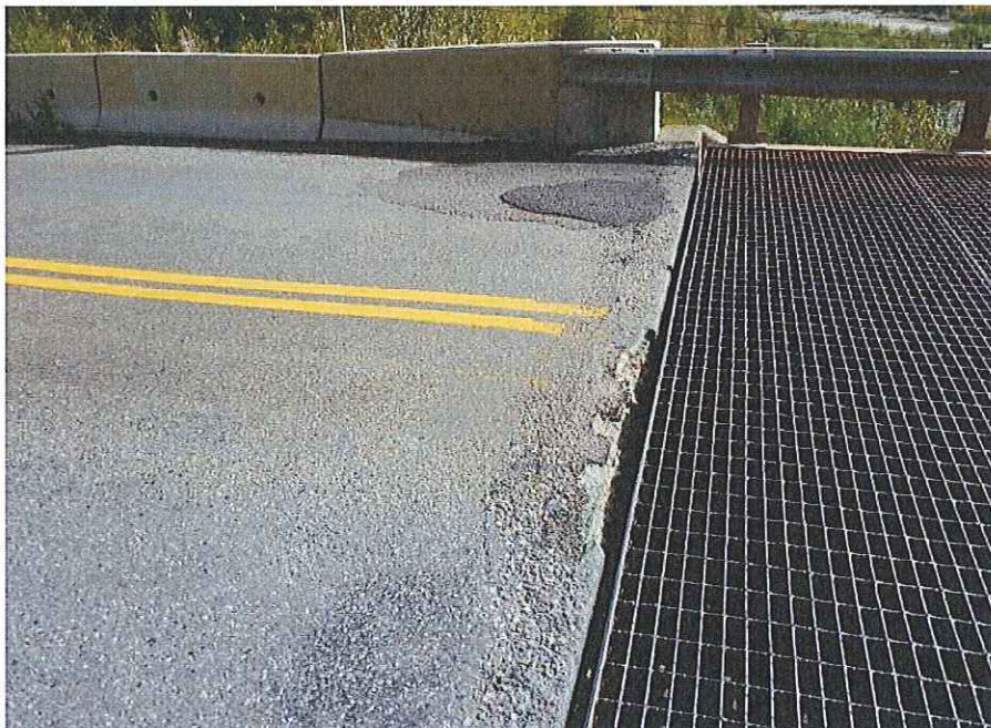
P50 - Damaged BST at N Abutment deck joint
