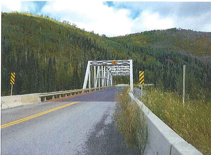
P58 - Missing stream ID sign on S approach
