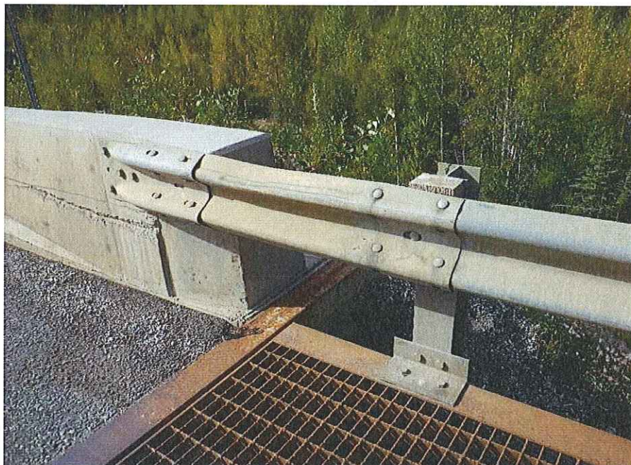
P54 - Incorrectly lapped W-beam railing at W side of S Abutment
