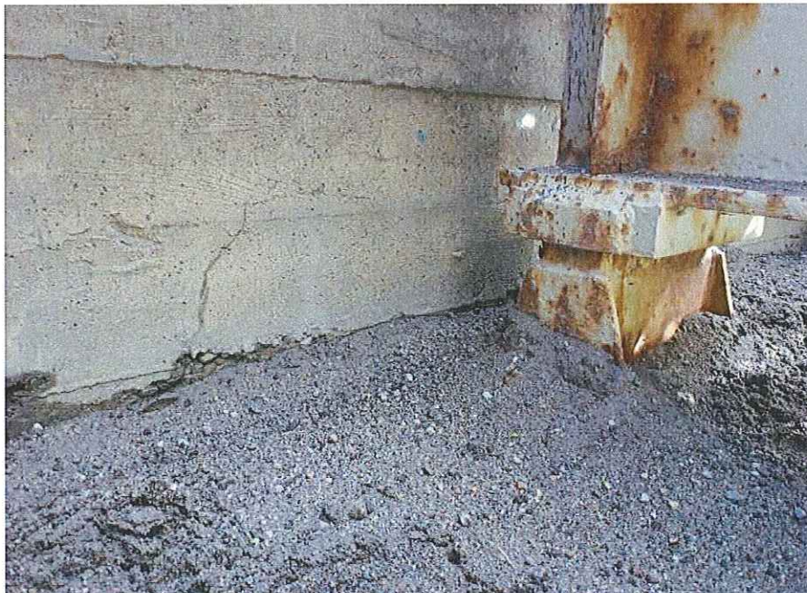
P42 - Typical debris on N Abutment bearing seat
