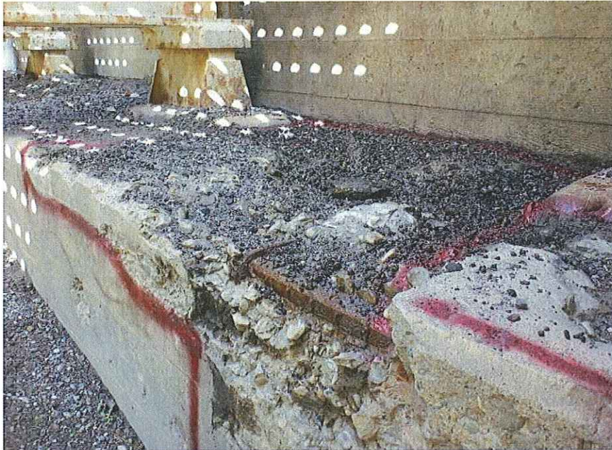
P41 - Spall with exposed rebar on N Abutment bearing seat
