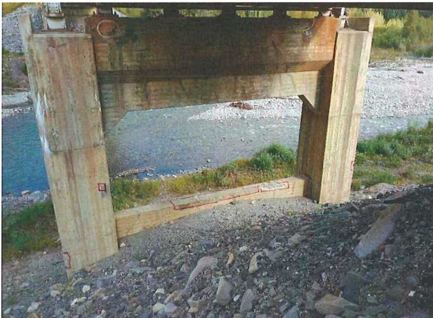
P20 - Delaminations on S Pier facing N from S Abutment
