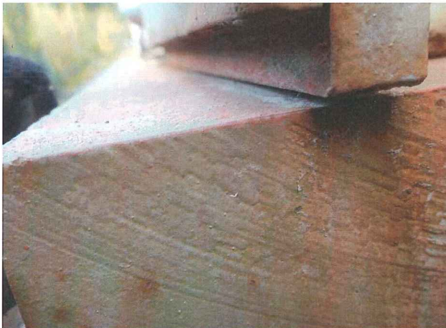
P36 - Gap between W flange on end post and bearing top plate at S end of W truss
