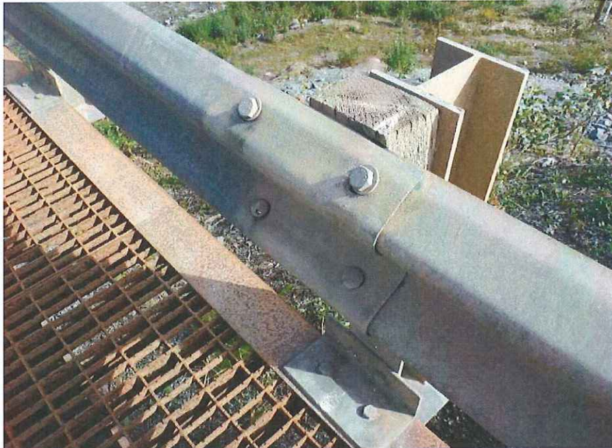
P55 - Hex head bolts in W-beam railing
