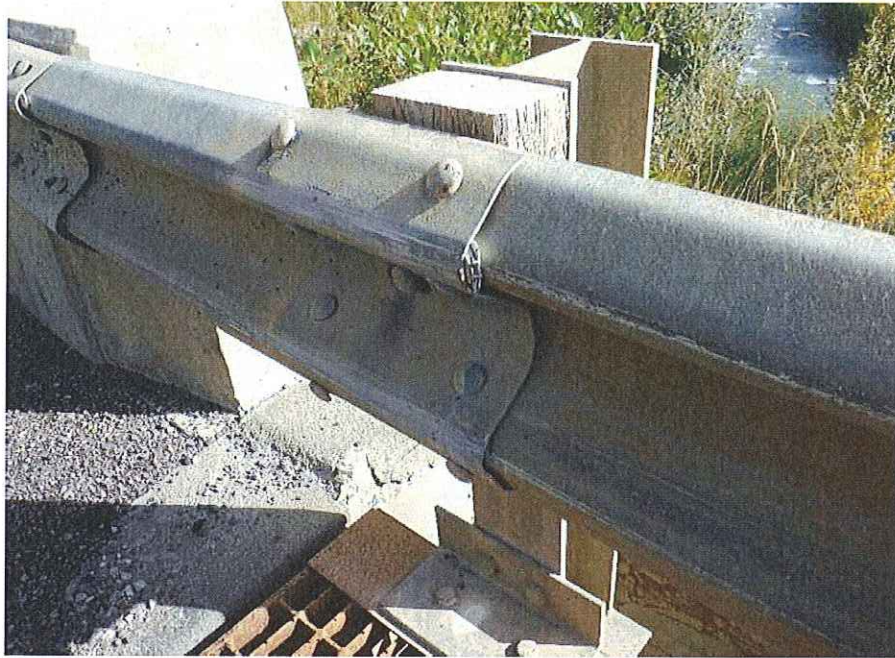
P53 - Incorrectly lapped W-beam railing at E side of N Abutment
