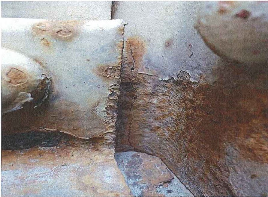
P33 - Cracking in steel at w side of end post at N end of W truss
