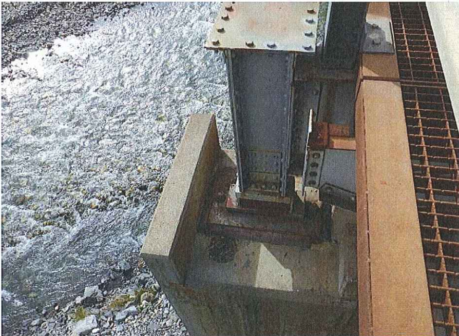
P30 - General view of end post on N end of E truss
