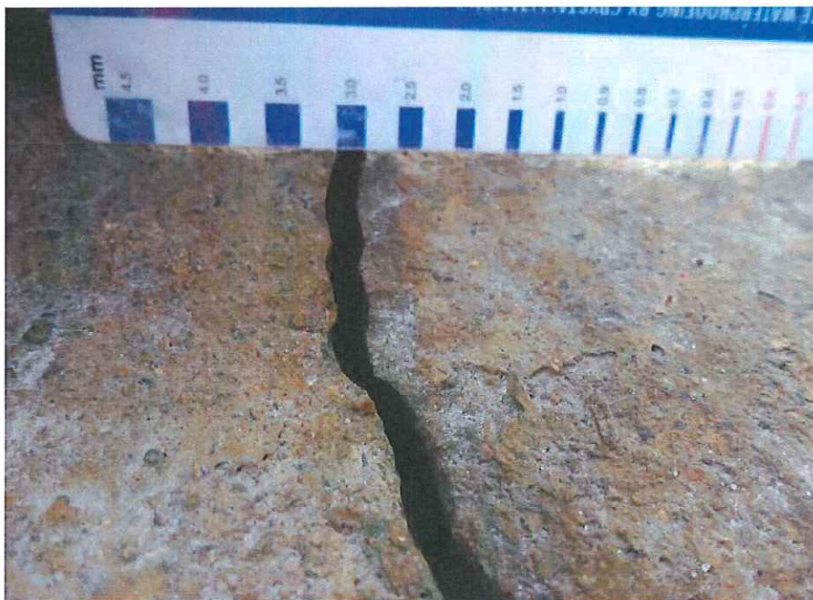
P28 - Wide vertical crack in middle of wall at base of N Pier
