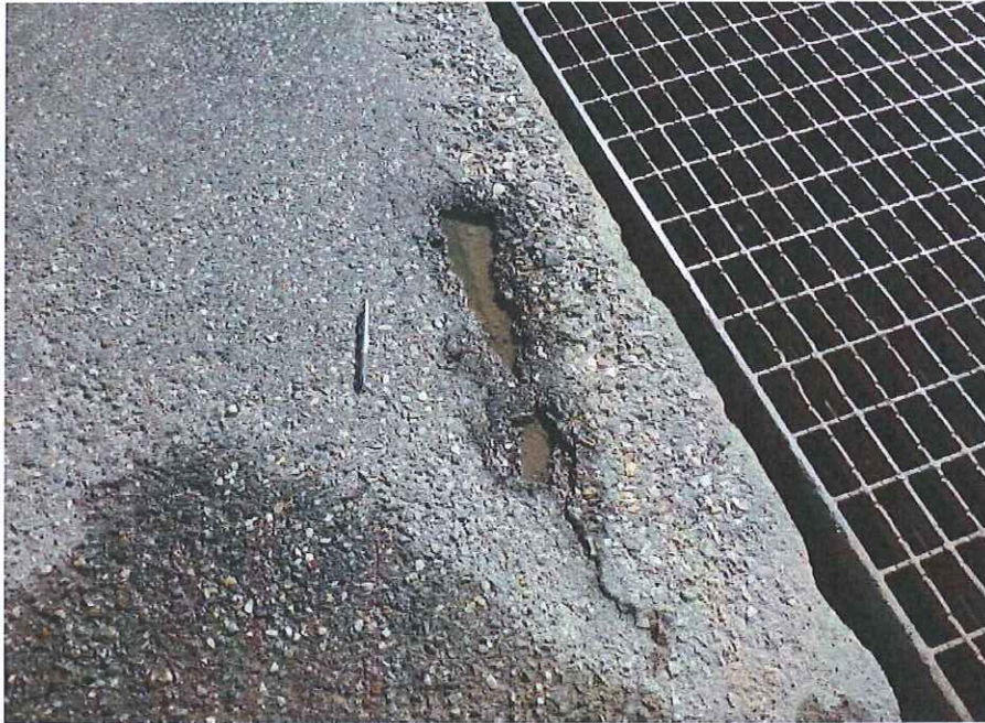
P51 - Damaged BST at N Abutment deck joint
