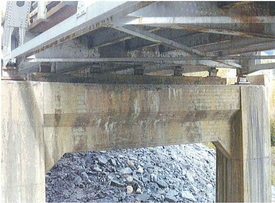
P25 - Spalls and leaching cracks on S face of N Pier
