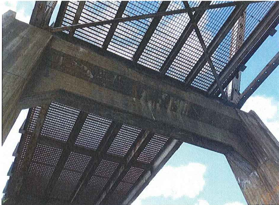
P21 - Leaching cracks and spalls on S Pier cap beam
