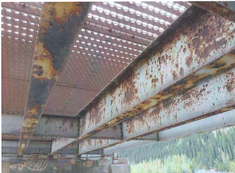
P56 - Typical condition of steel coating on Span 3 girders
