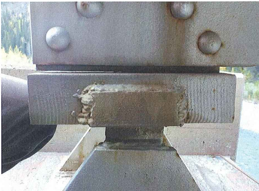
P34 - Gap between E flange on end post and bearing top plate at S end of W truss
