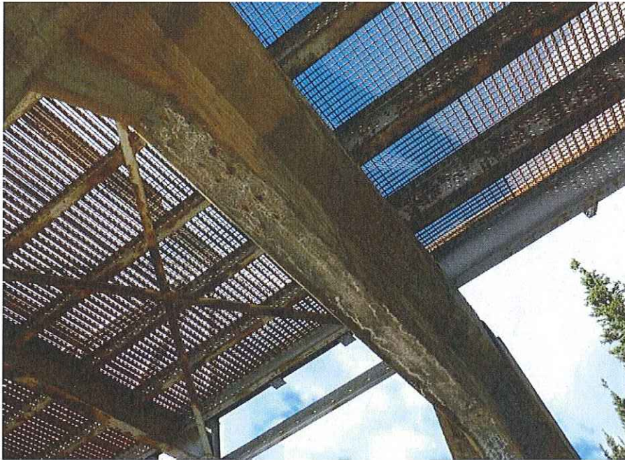
P29 - Efflorescence, cracking and scaling on soffit of N Pier cap beam
