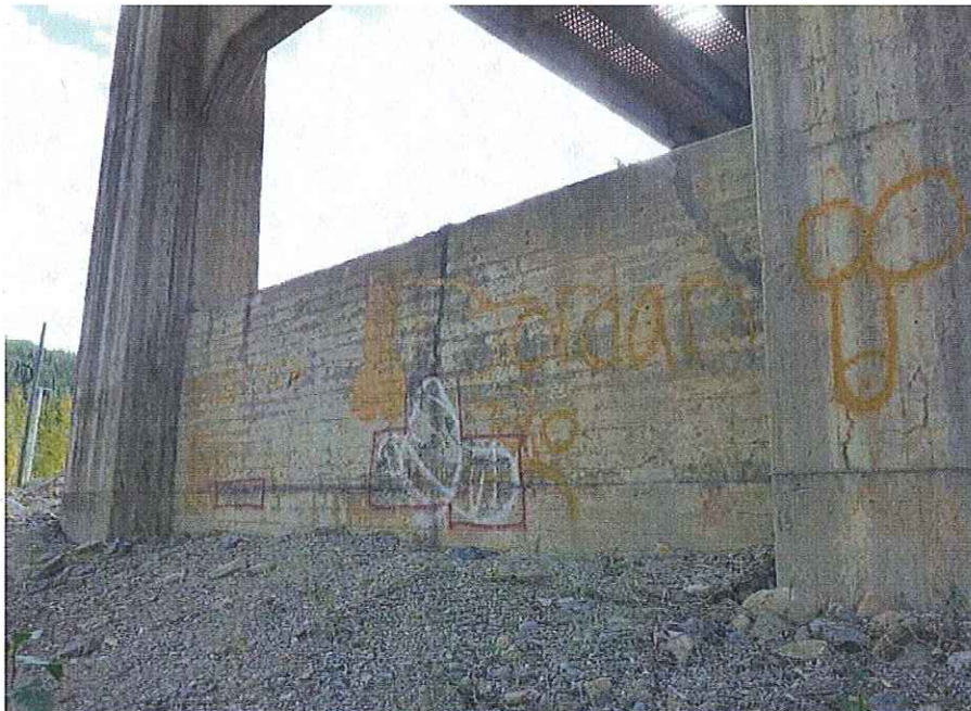
P22 - Delaminations on N face of wall at base of S Pier
