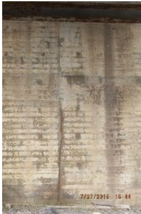
Photo 6 – Wide vertical crack pier 2 of the Tetsa structure, with rust staining from corroded rebar within.
