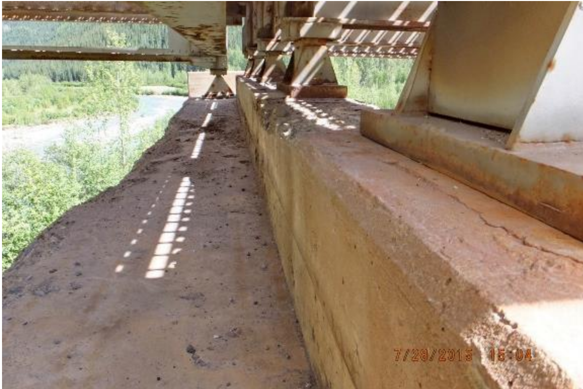
Photo 2 – MacDonald Bridge, south pier cap, spalls near bearings.
