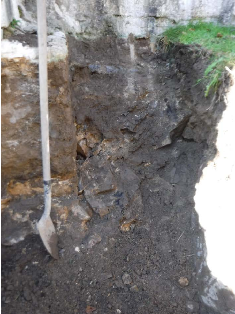
Test Pit #3 – Grouted rubble at base of chamber wall
