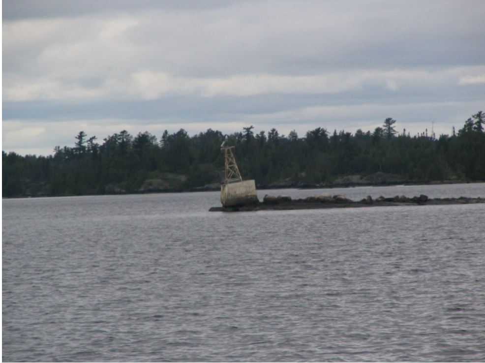
Figure 5: Existing Navaid, and Deteriorated Foundation (to be removed)
