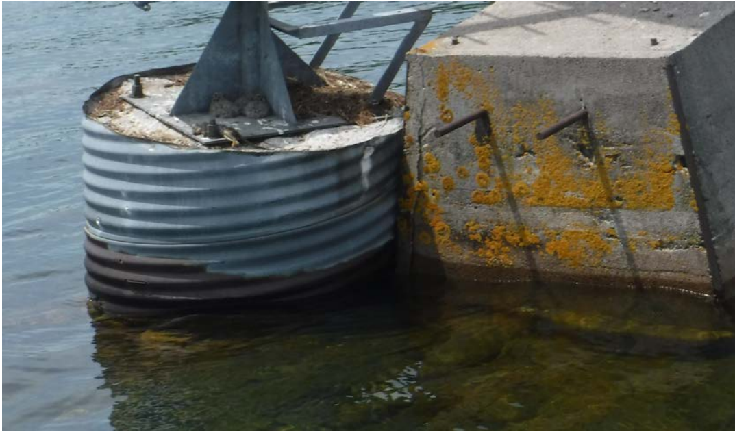
Figure 6: Existing Weathered Piers (To be Removed)
