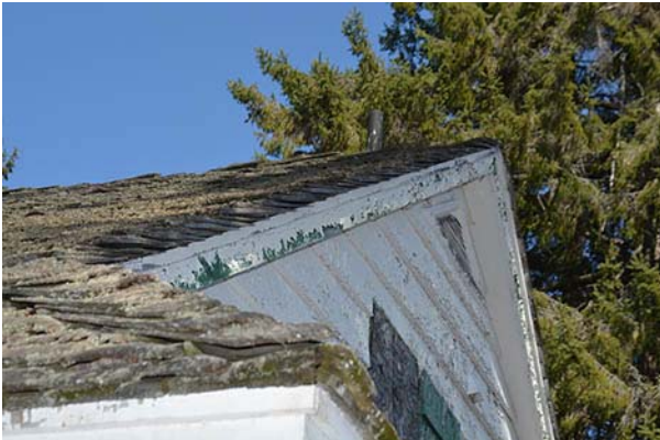
Image 13: The trim and accent colours were previously green, but some areas have been painted over with white. Source: HCS, 2017
