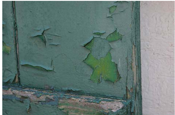
Image 12: The “mossy” green paint layer is visible underneath the current green. Source: HCS, 2017
