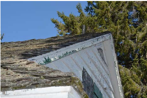
Image 13: The trim and accent colours were previously green, but some areas have been painted over with white. Source: HCS, 2017
