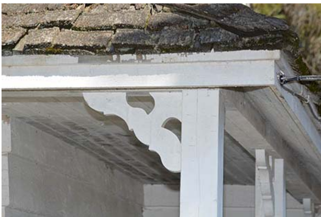
Image 7: The simple detailing, as expressed in the limited decorative elements, such as the shutters and verandah roof brackets. Source: HCS, 2017
